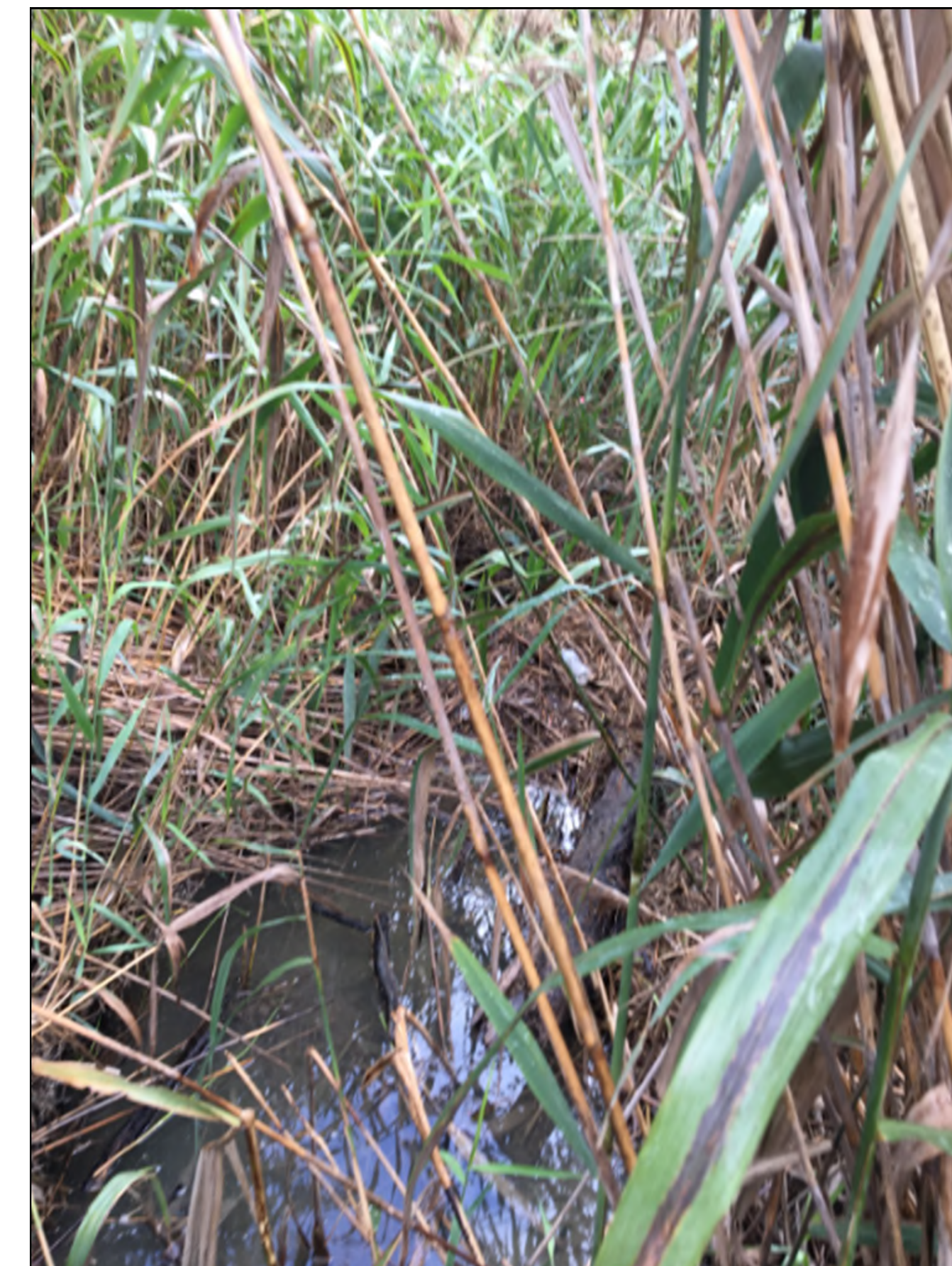
PARTIAL BLOCKAGE IN DRAIN
