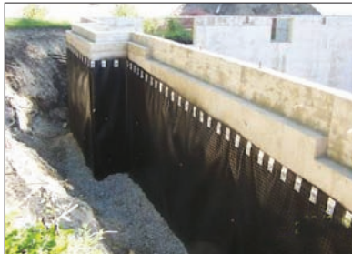
A gap around the basement wall in a home that is under construction.
