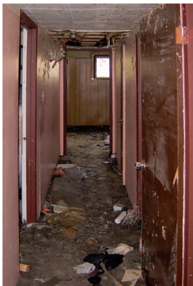
Finished basements experience far greater damages than unfinished basements when the basement floods.
