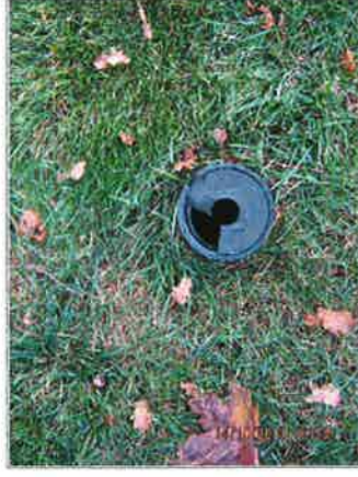
DAMAGED CLEANOUT CAPS
