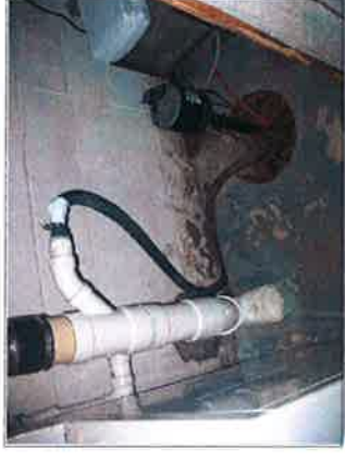
SUMP PUMP CONNECTED TO A SANITARY DRAIN CONNECTION
