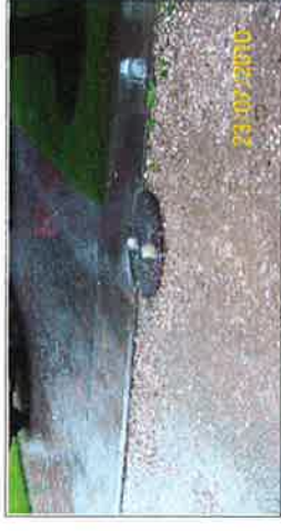
STORM SEWER SURCHARGE ESCAPING MANHOLE COVER
