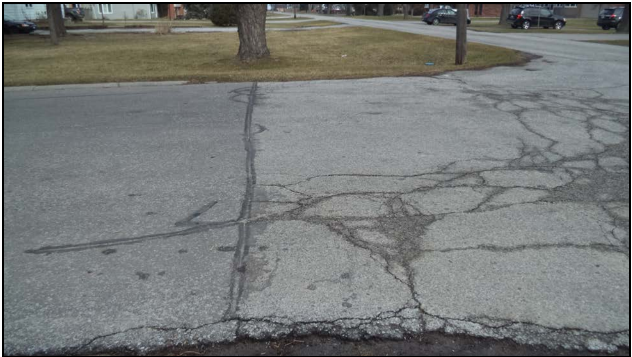
Photograph 8 – Wearing Surface at West Approach
