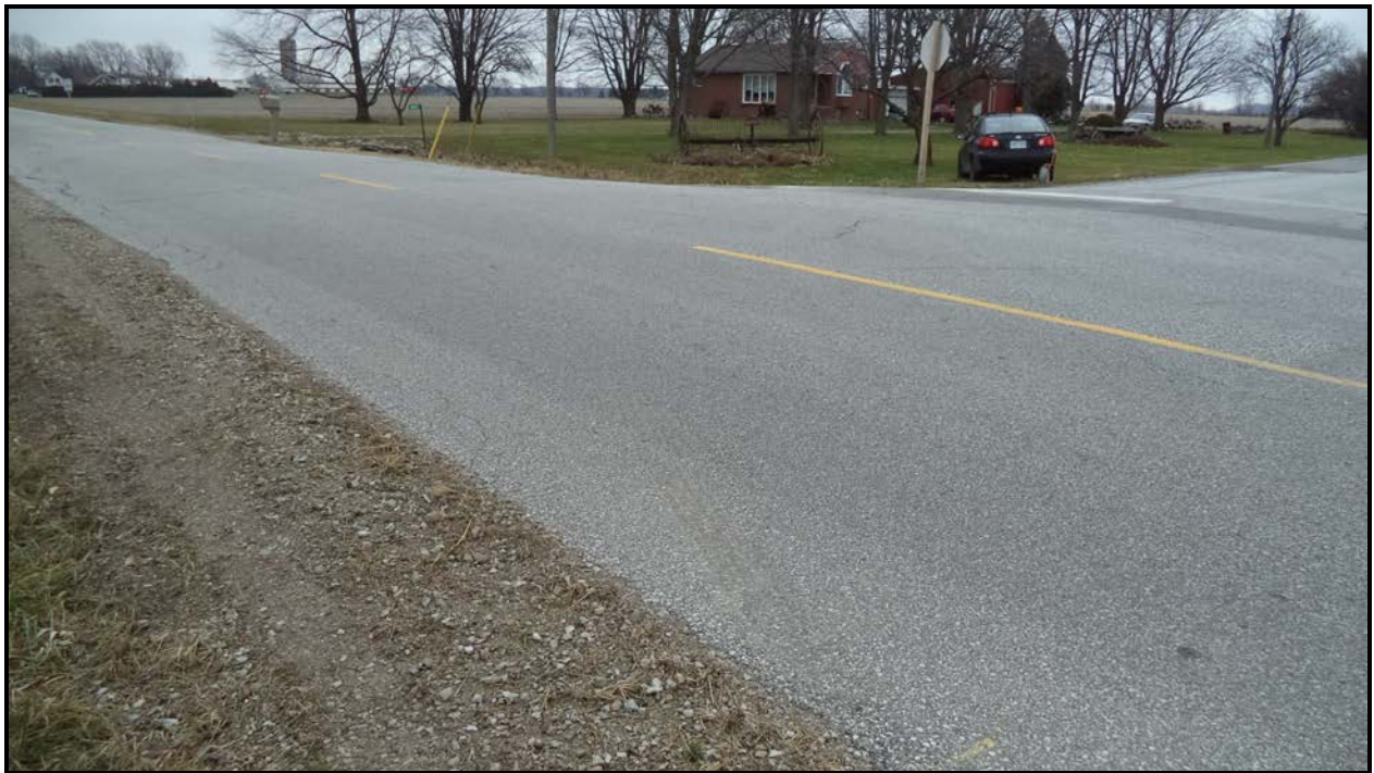
Photograph 6 – Wearing Surface at West Approach
