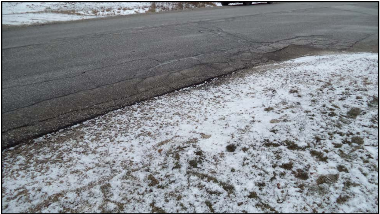
Photograph 6 – Wearing Surface at East Approach (Looking East)
