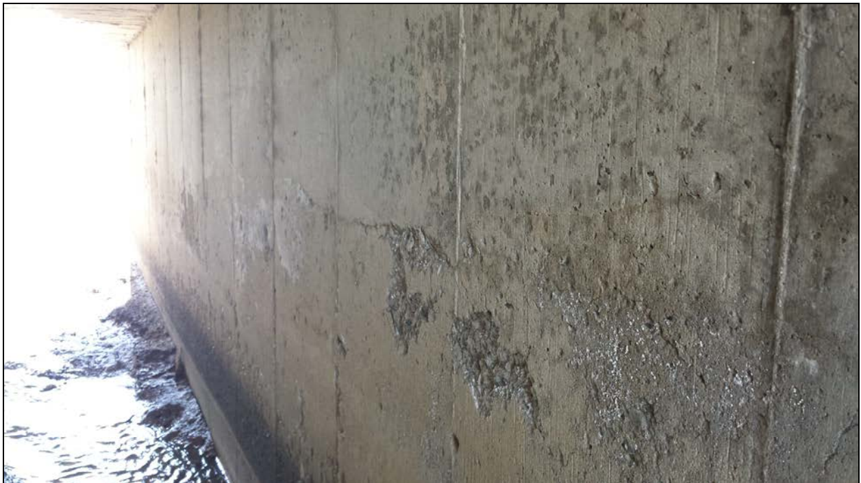
Photograph 4 – Typical scaling and honeycombing at both walls
