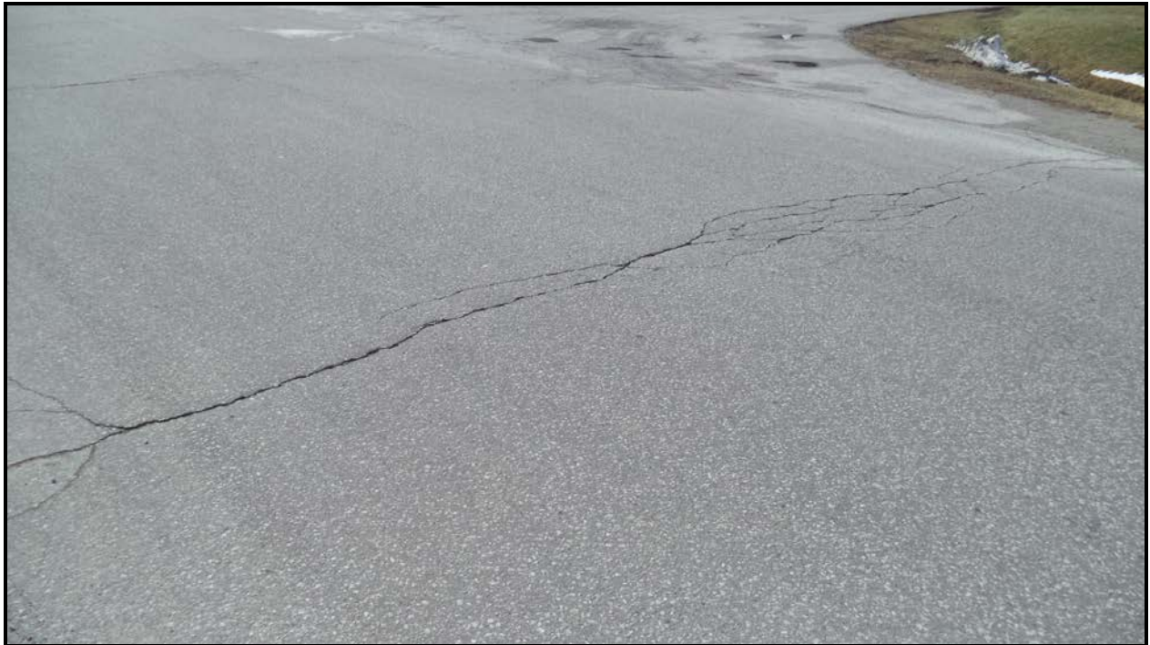
Photograph 5 – Wearing Surface at West Approach
