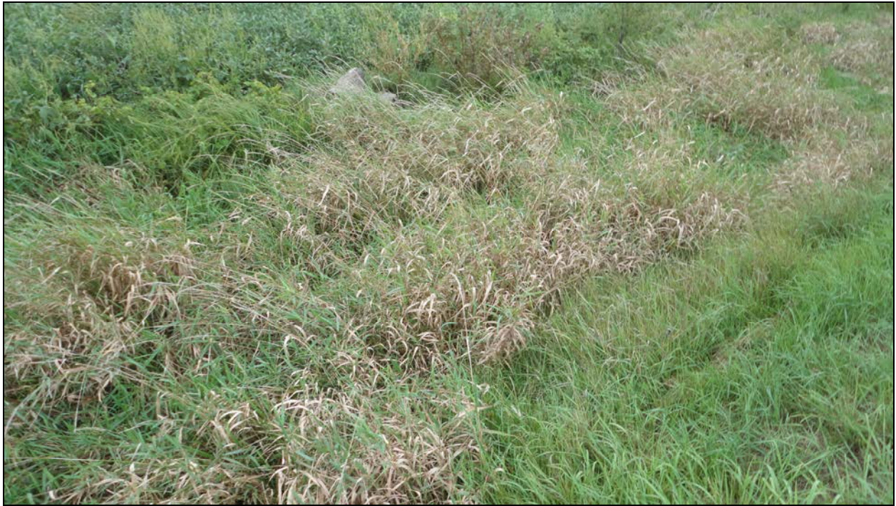
Photograph 5 – Heavy Plants Growth at East Elevation (Looking East)
