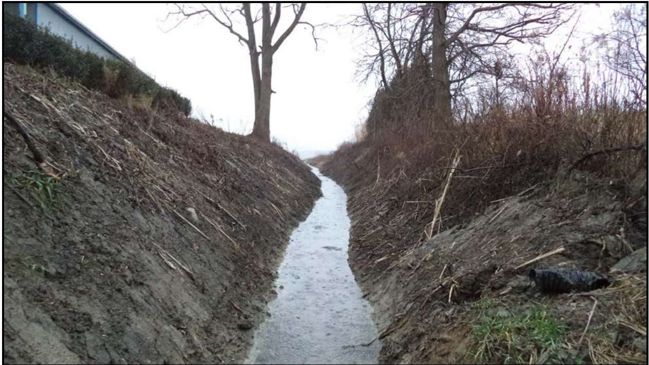
Photograph 7 –Water Stream (Snake Lane Road West Side – Looking East)
