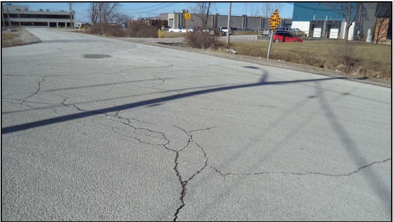
Photograph 6 – Wearing Surface at West Approach
