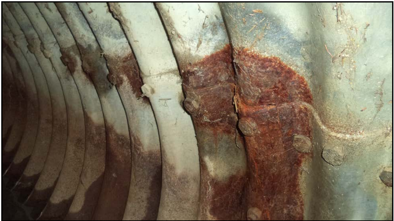
Photograph 4 – Culvert haunches corrosion
