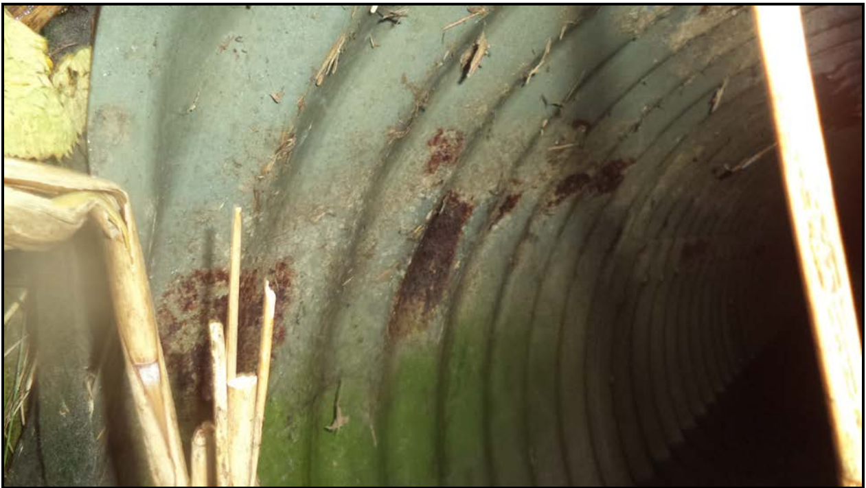
Photograph 4 – Culvert Barrel Side Corrosion
