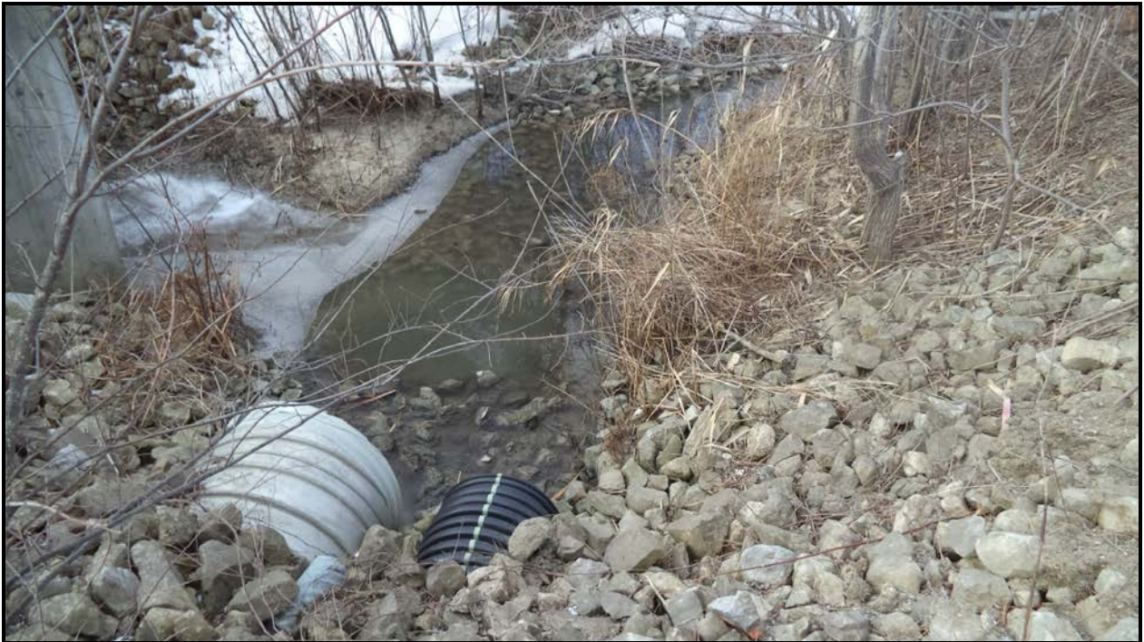
Photograph 7 – Water Stream (Outer Drive West Side – Looking West)
