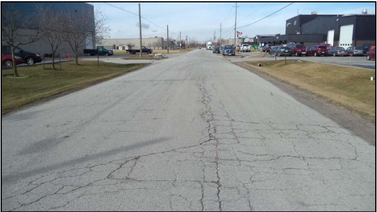
Photograph 6 – Wearing Surface at West Approach
