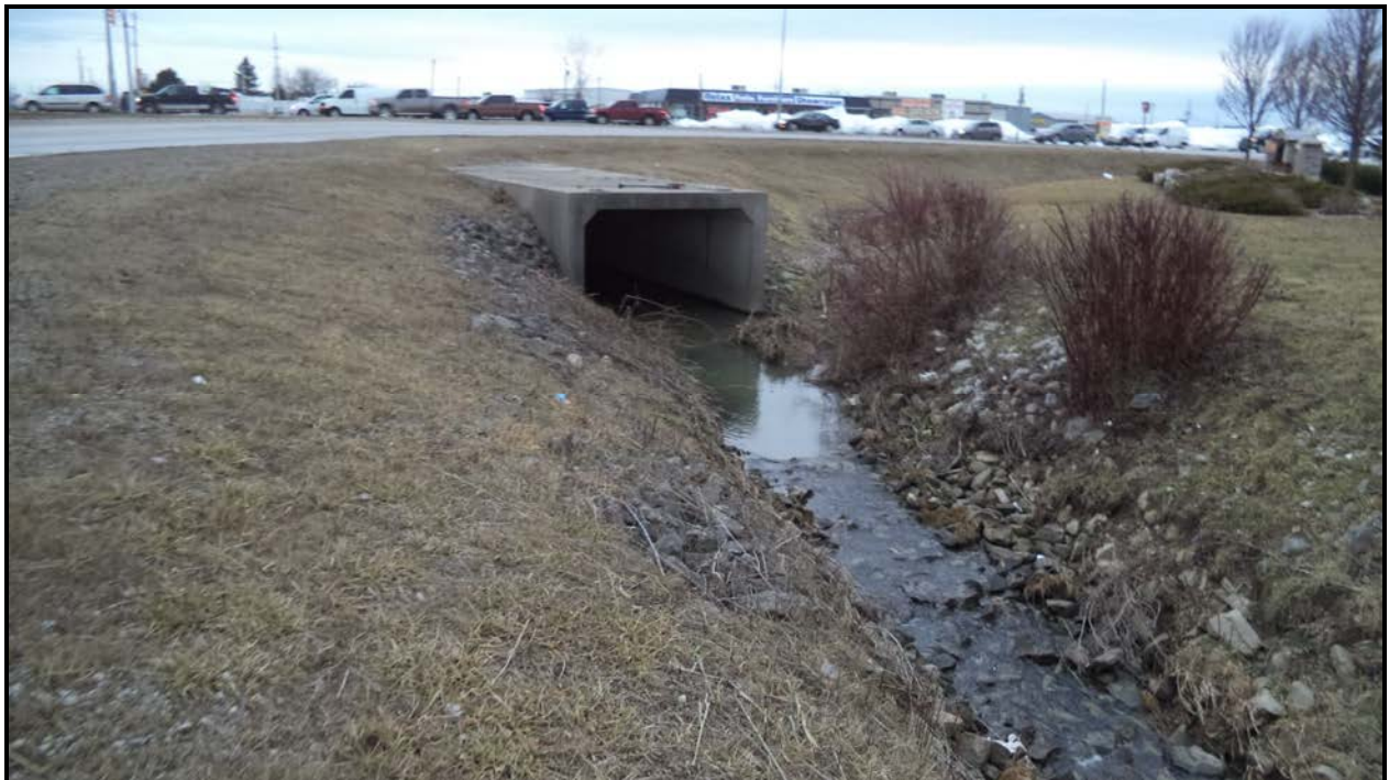
Photograph 4 – Water Stream (Manning Road West Side - Looking South)
