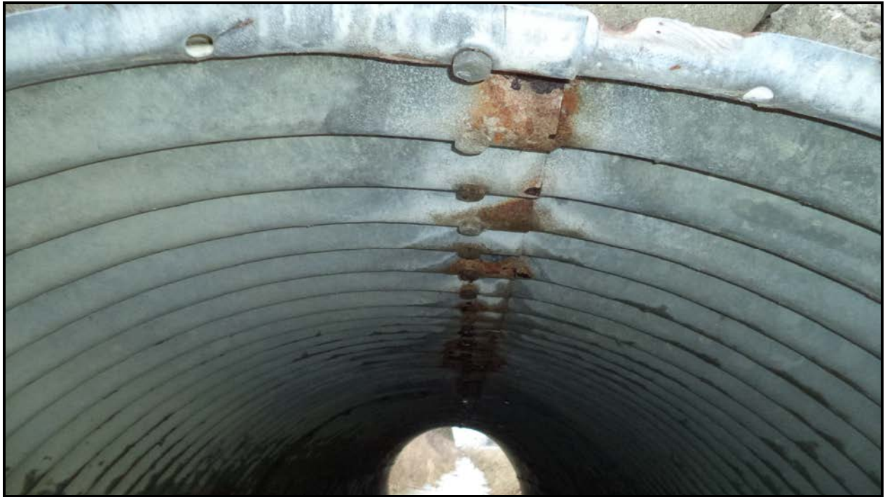
Photograph 3 – Bolts Corrosion at Culvert Soffit
