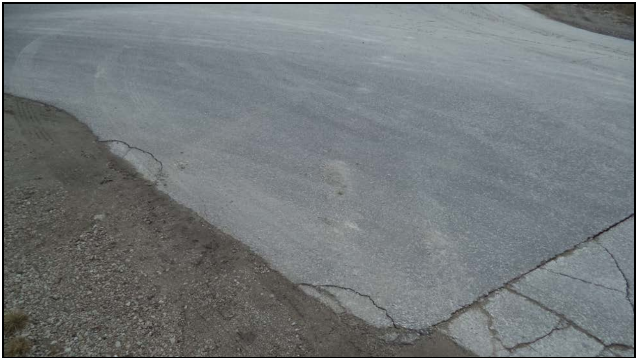
Photograph 8 – Wearing Surface at West Approach
