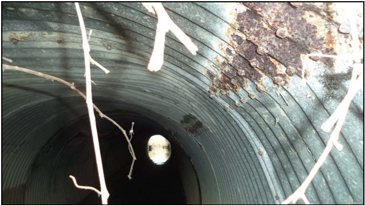
Photograph 4 – Typical Corrosion at Bolted Connections
