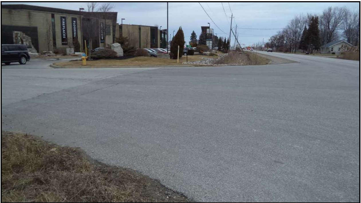
Photograph 6 – Wearing Surface at West Approach
