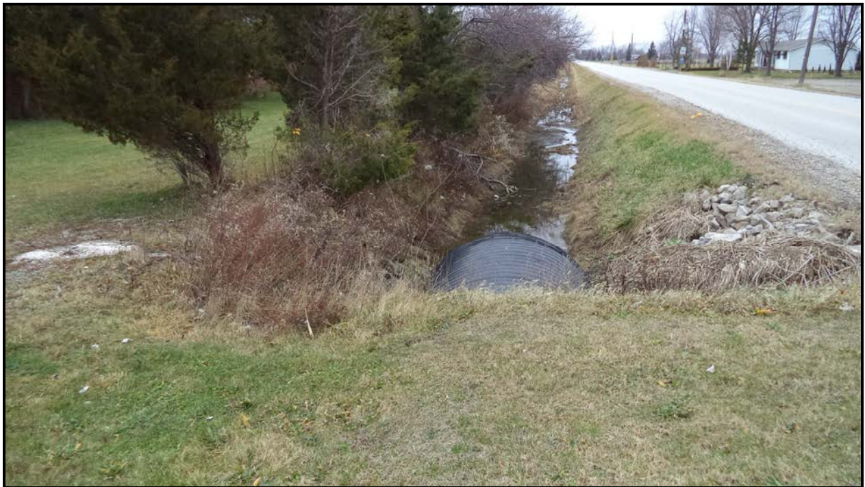
Photograph 8 – Water Stream (Malden Road East Side – Looking West)
