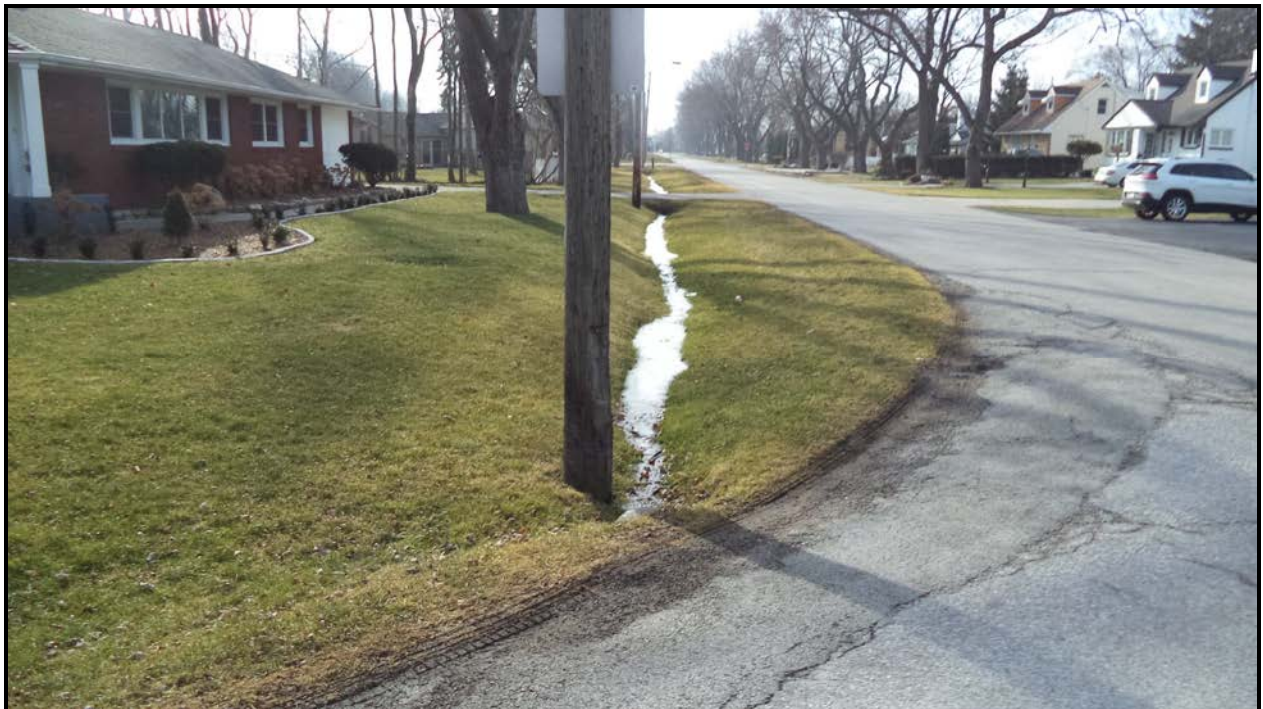
Photograph 8 – Water Stream (Arlington Blvd. Road East Side - Looking South)
