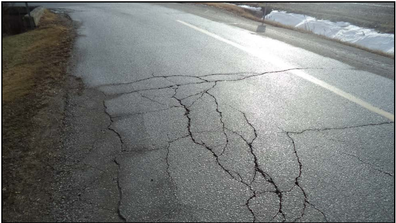
Photograph 6 – Wearing Surface at West Approach
