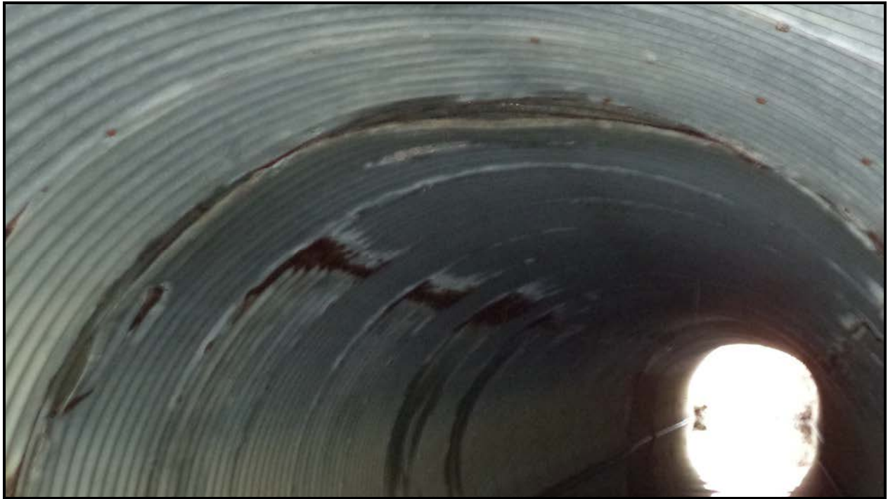
Photograph 3 – Bending and Settlement at the Barrel Top
