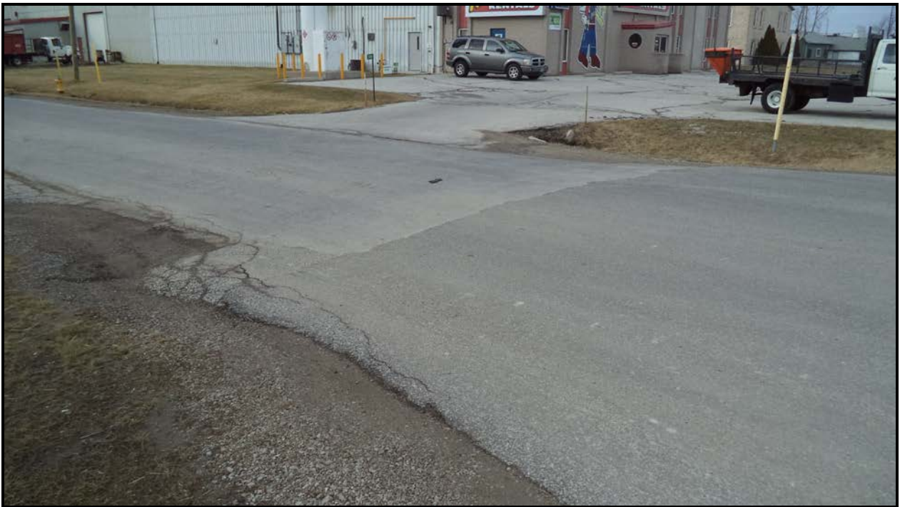
Photograph 8 – Wearing Surface at West Approach
