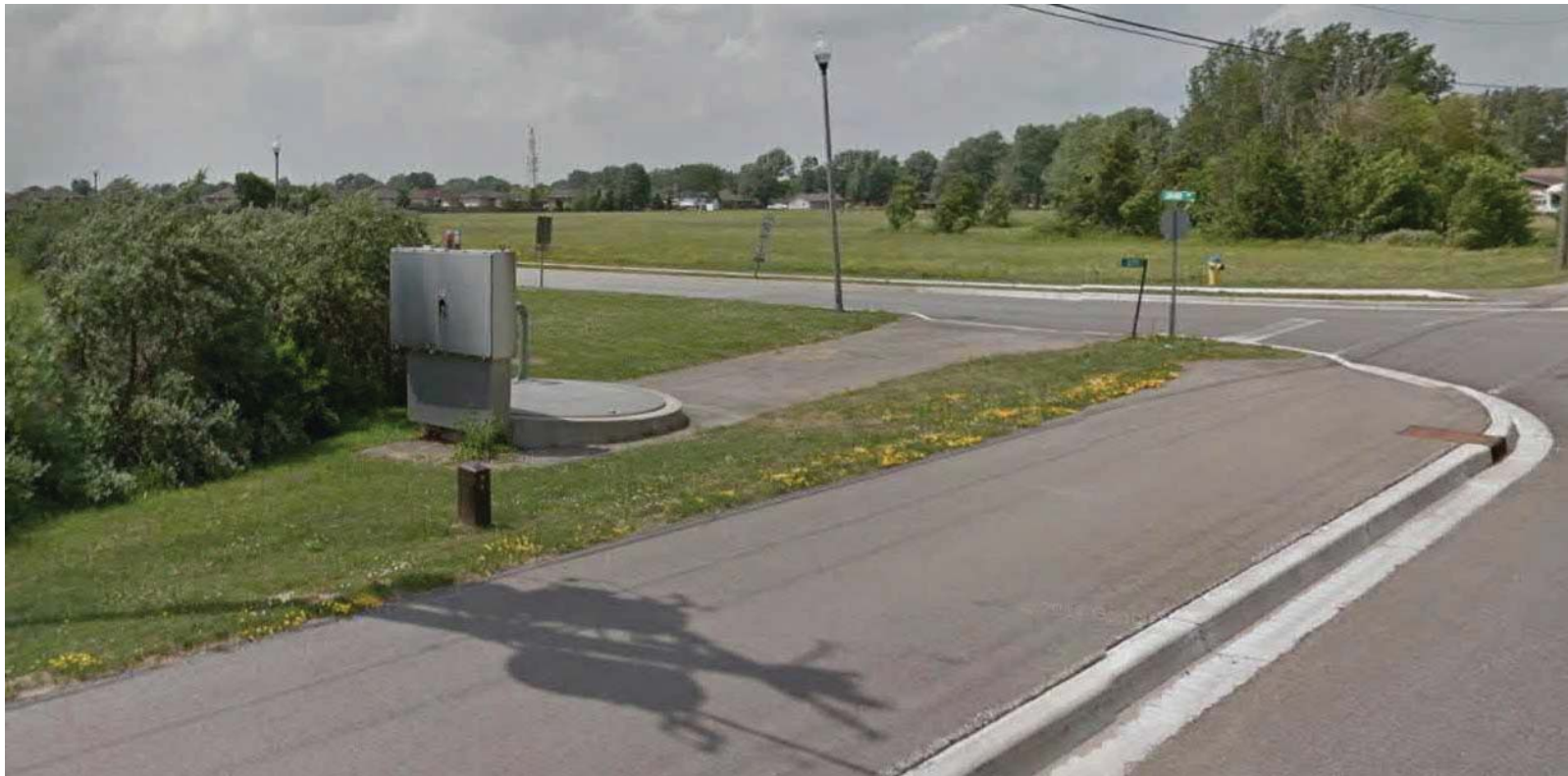
EXAMPLE OF A PUMP STATION ELECTRICAL BOX
