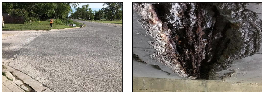
Figure 3: Asphalt over steel plate repair on deck top (left), typ. soffit deterioration (right)
