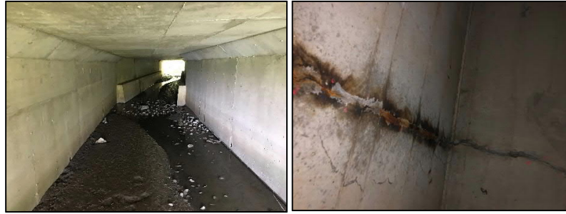
Figure 5: Culvert barrel (left), typ. soffit deterioration (right)
