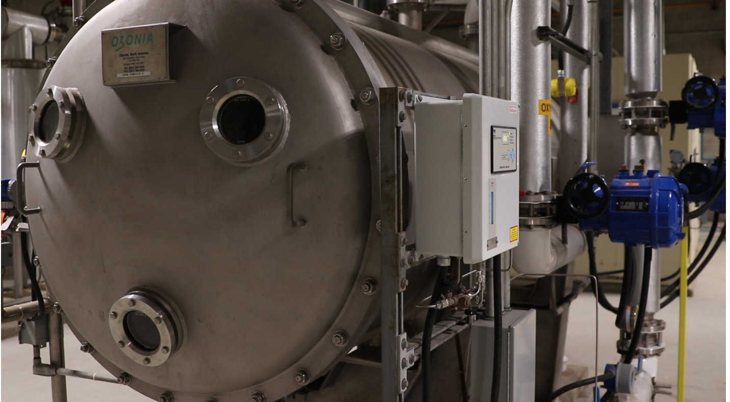
Ozone Generator at the A.H. Weeks Water Treatment Plant
