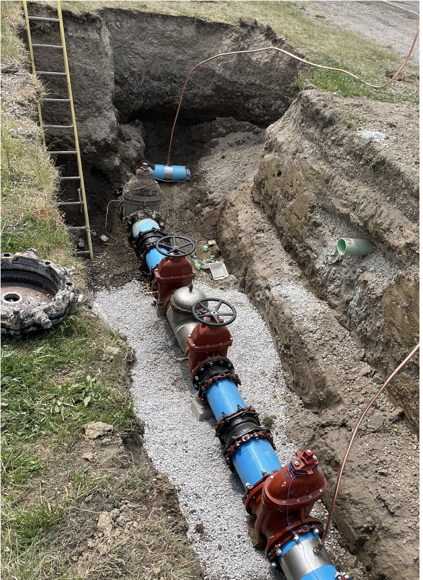
Water source to fill the 1050 mm feedermain using a 250 mm backflow preventer
