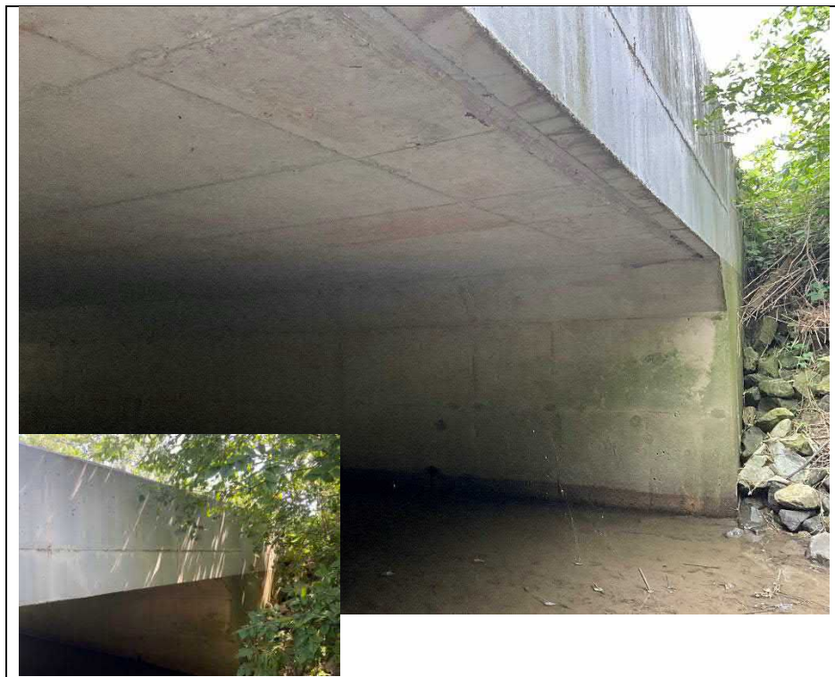
Photograph 8: West elevation with typical cracking at headwalls with efflorescence
