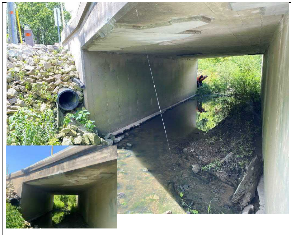
Photograph 6: Concrete soffit patch at east end of soffit
