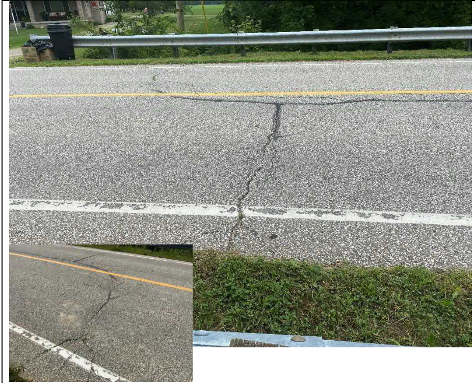
Photograph 3: Wearing surface over the structure with transverse crack (Looking West)
