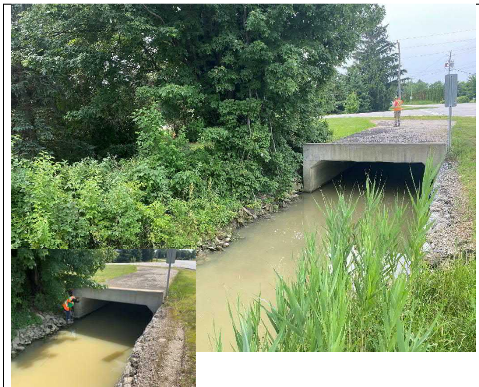
Photograph 8: North inlet with exposed waterproofing along the top of deck (Looking South)
