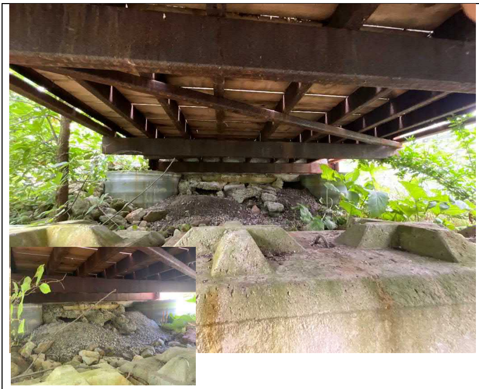
Photograph 10: Concrete caissons at north end with void under approach slab
