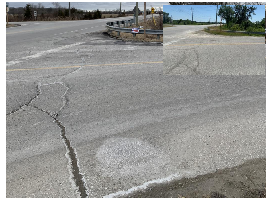
Photograph 2: Wide crack at joint between wearing surface over the culvert and the east approach
