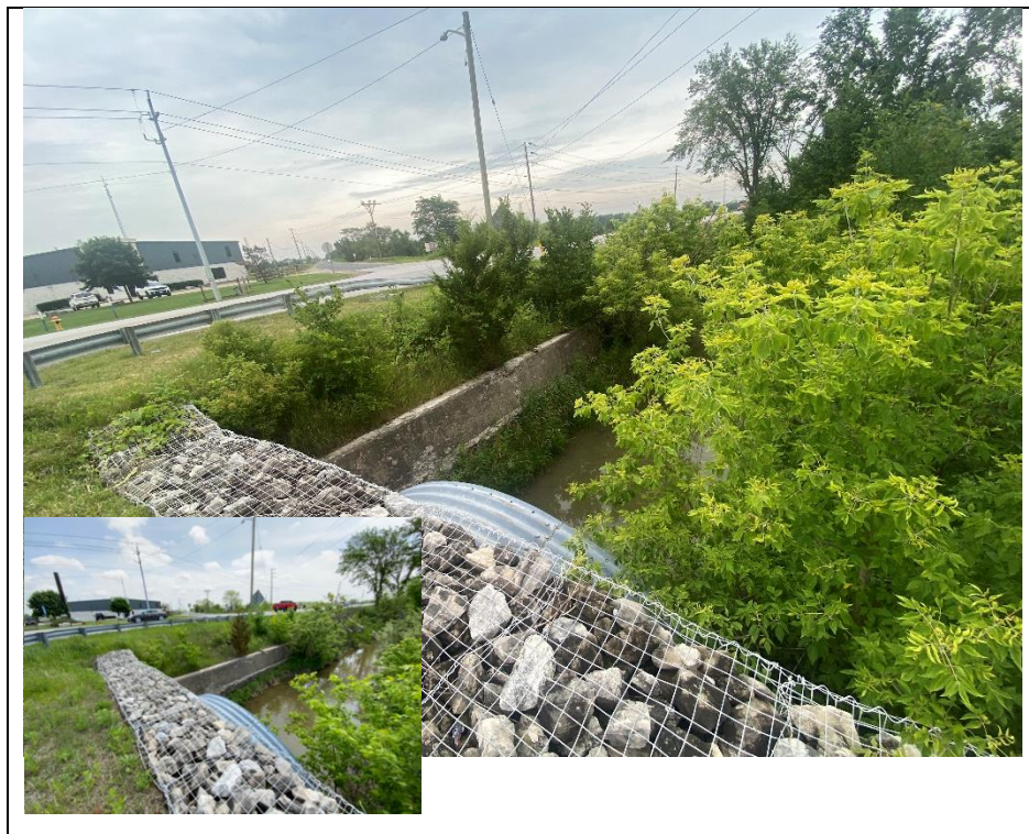
Photograph 16: Retaining wall, gabion baskets, and culvert end at south elevation (Looking East). Note: The retaining wall is part of the drain which is attributed to the county road.
