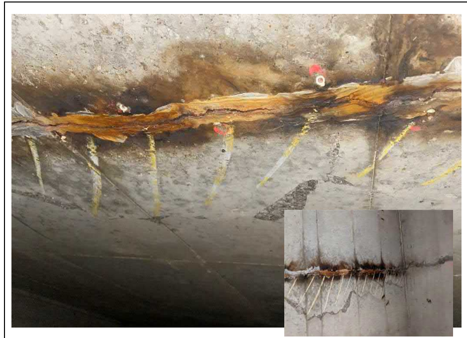
Photograph 12: Typical delamination, and epoxy injected cracks with staining along soffit within the original section of the culvert
