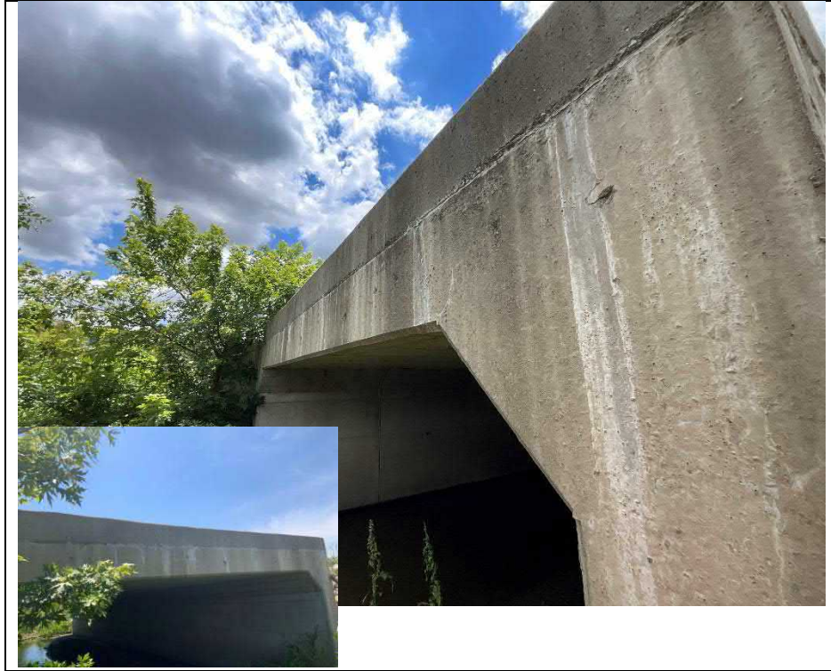
Photograph 9: Discrete locations of light spalling at the south headwall
