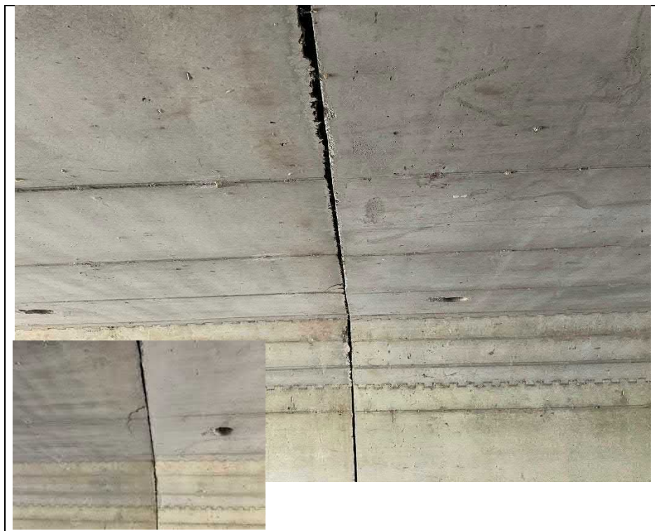
Photograph 12: Typical delamination on soffit at joints between precast units
