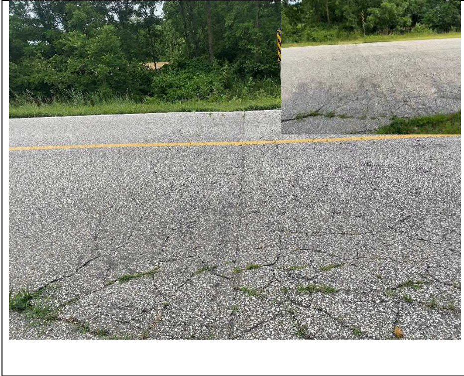
Photograph 3: Cracking of asphalt pavement at interface of deck and south approach (Looking East)
