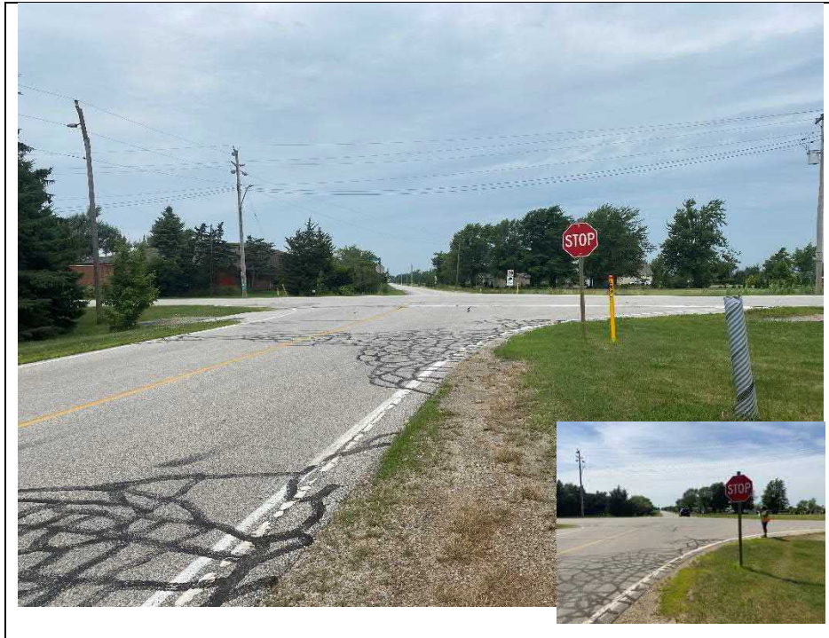
Photograph 1: Wearing surface over structure (Looking West). Cracks have been sealed since the last inspection
