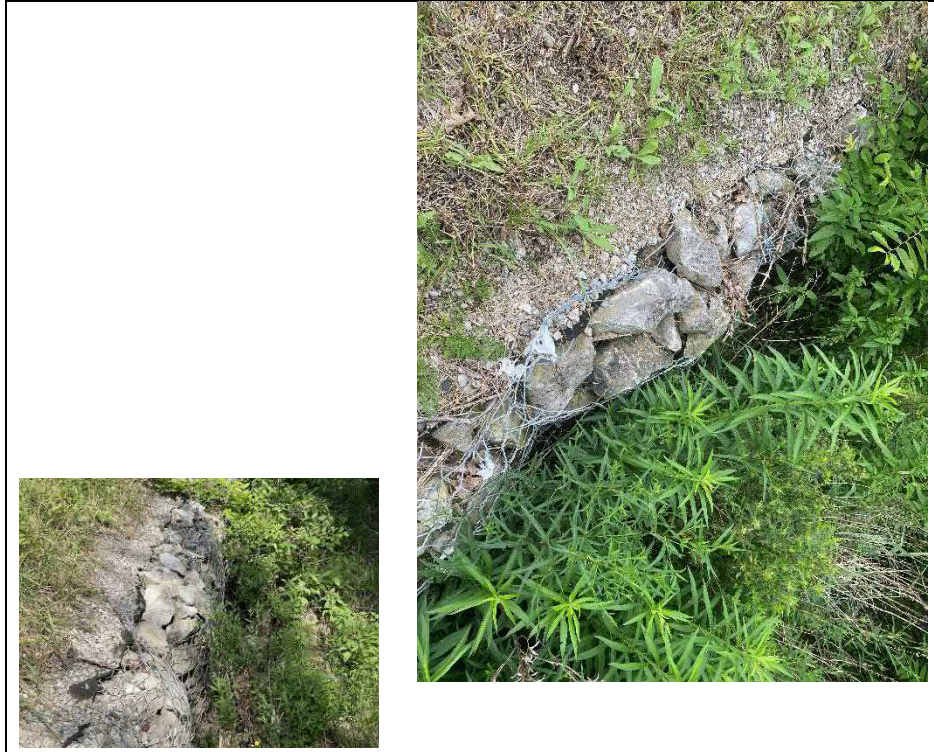
Photograph 13: Ruptured gabion basket at west embankment
