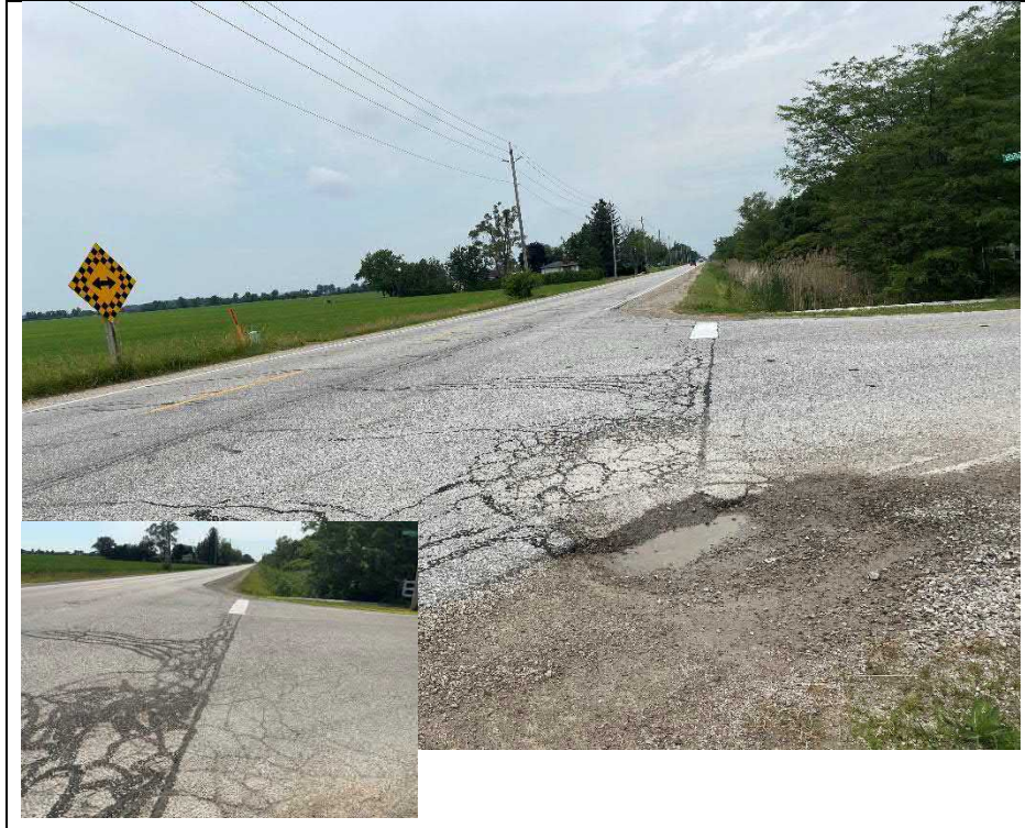
Photograph 3: Alligator cracking of wearing surface at southeast quadrant (Looking West)
