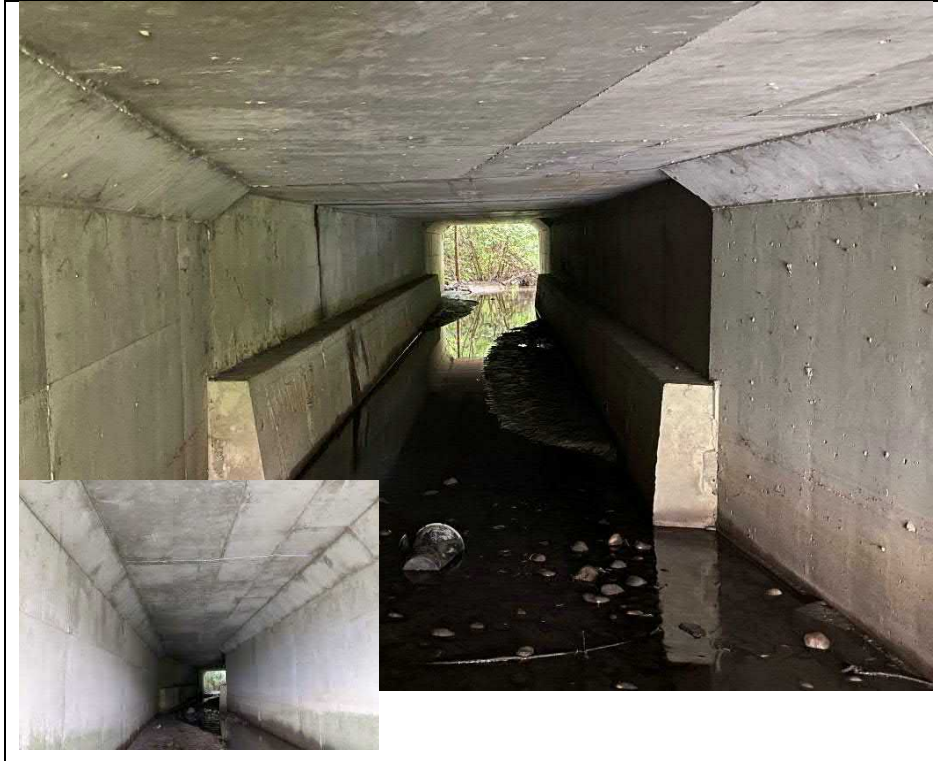
Photograph 11: Culvert barrel, showing the non-rigid original section of the culvert with jacketed footings, as well as the new rigid frame section extension (Looking Northwest)
