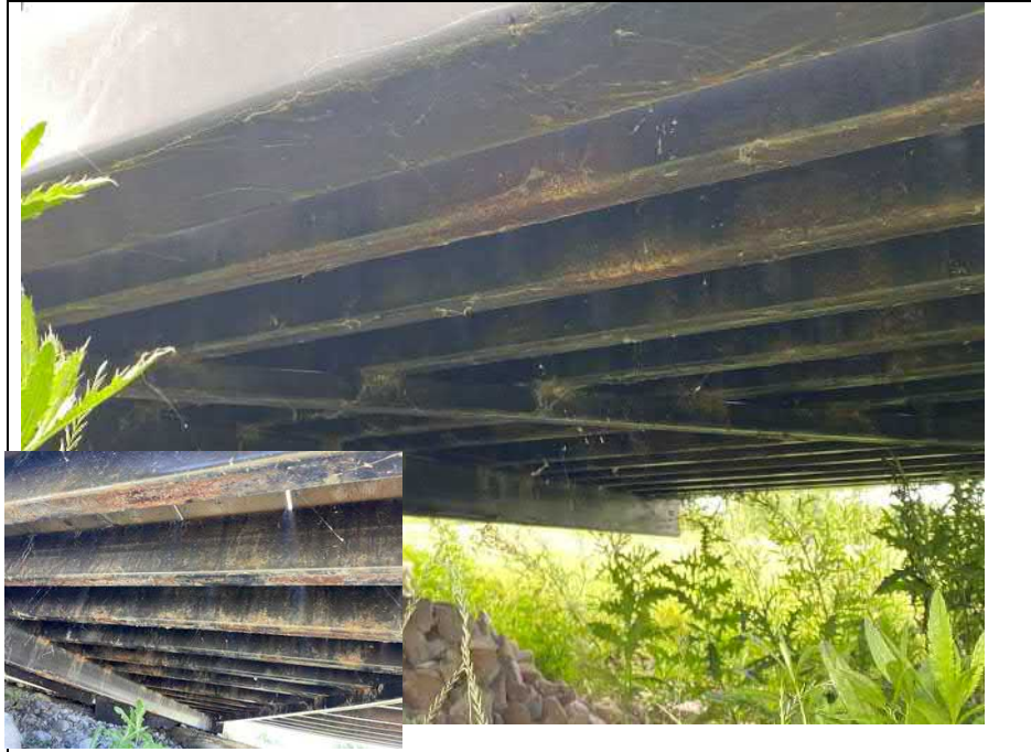
Photograph 11: Typical severe corrosion on several stringer members
