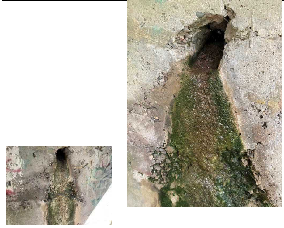
Photograph 15: Efflorescence and honeycombing on north abutment wall
