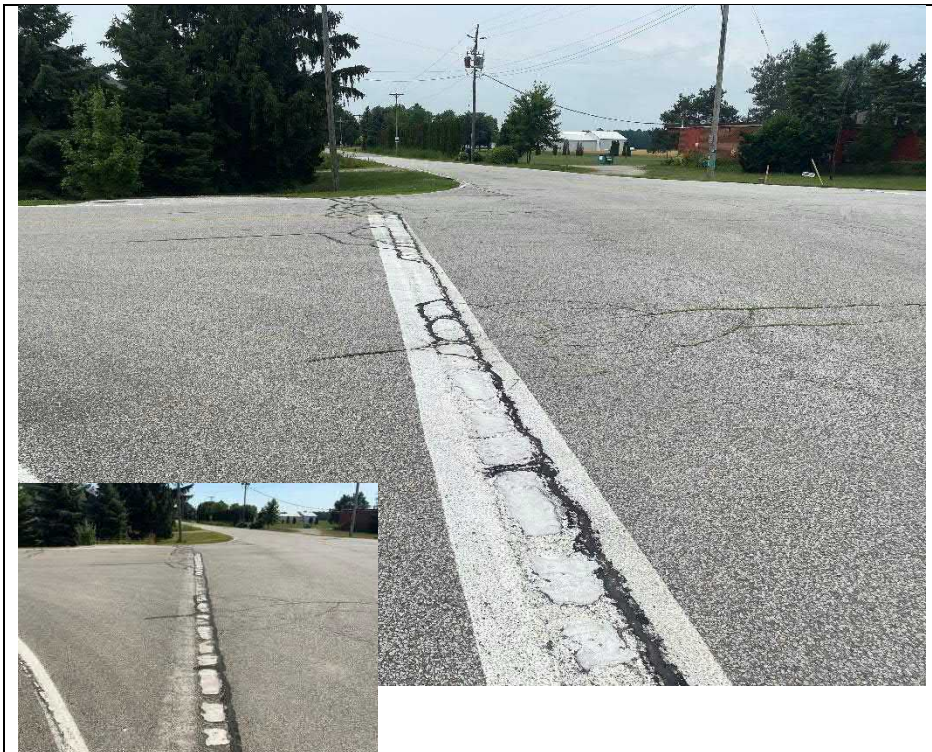
Photograph 4: Sealed wide cracks on the wearing surface at the west approach (Looking South)
