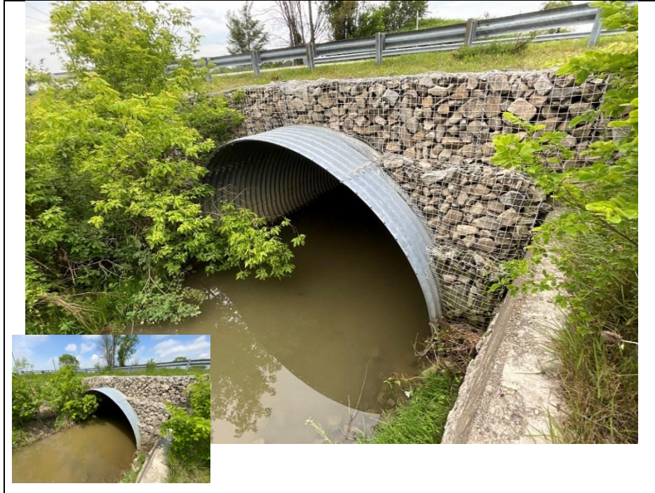
Photograph 9: South elevation with rip-rap slope protection, and gabion basket retaining walls (Looking North)
