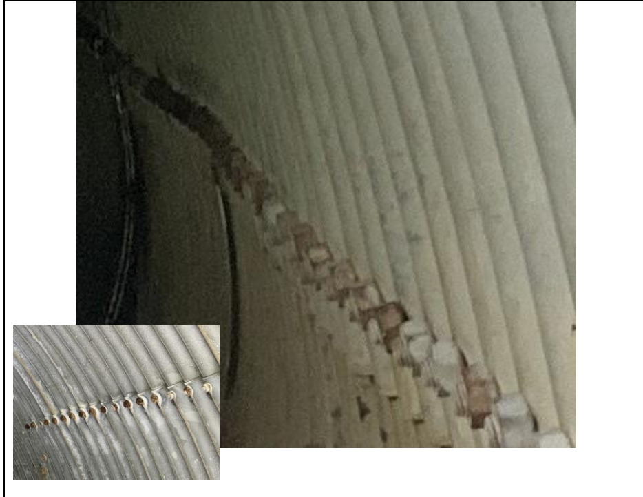
Photograph 13: Typical light to medium corrosion on bolts heads
