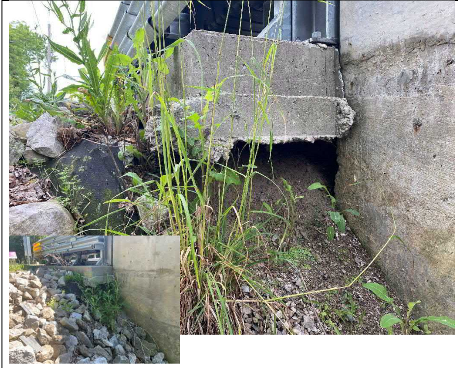
Photograph 13: Erosion below approach slab at the northwest wingwall
