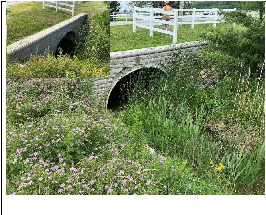
Photograph 4: East elevation with excessive vegetation (Looking North)
