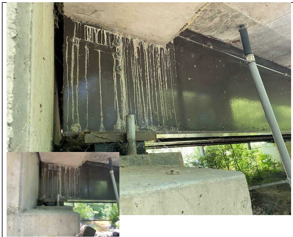
Photograph 12: Bearing seat at east abutment wall with typical bent anchor bolt (Looking South)
