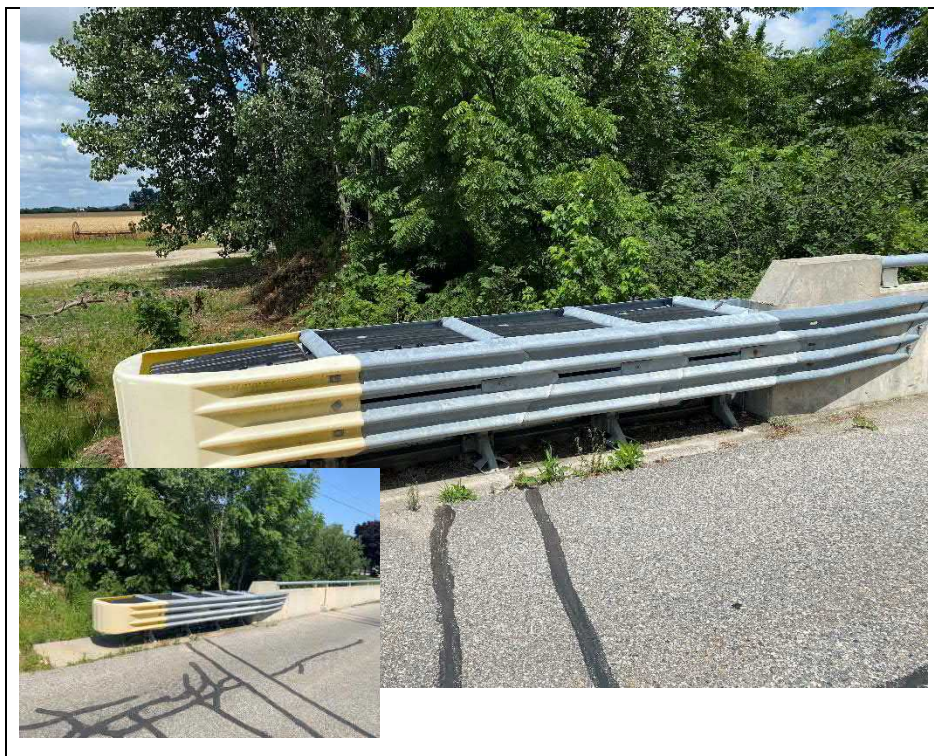
Photograph 12: Typical condition of energy attenuator at the southwest approach (Looking North)
