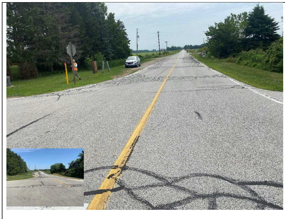
Photograph 2: Wearing surface over structure (Looking East). Cracks have been sealed since the last inspection
