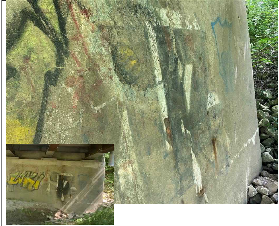
Photograph 19: Medium crack with active wet areas and efflorescence at north abutment wall
