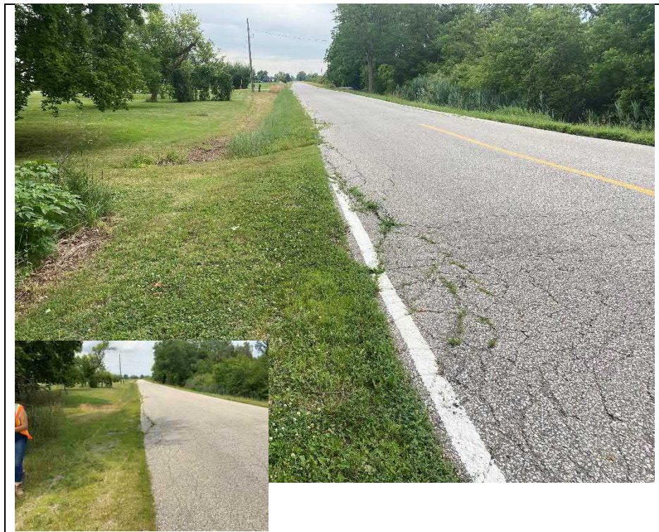
Photograph 4: Edge cracking of wearing surface at north approach (Looking North)
