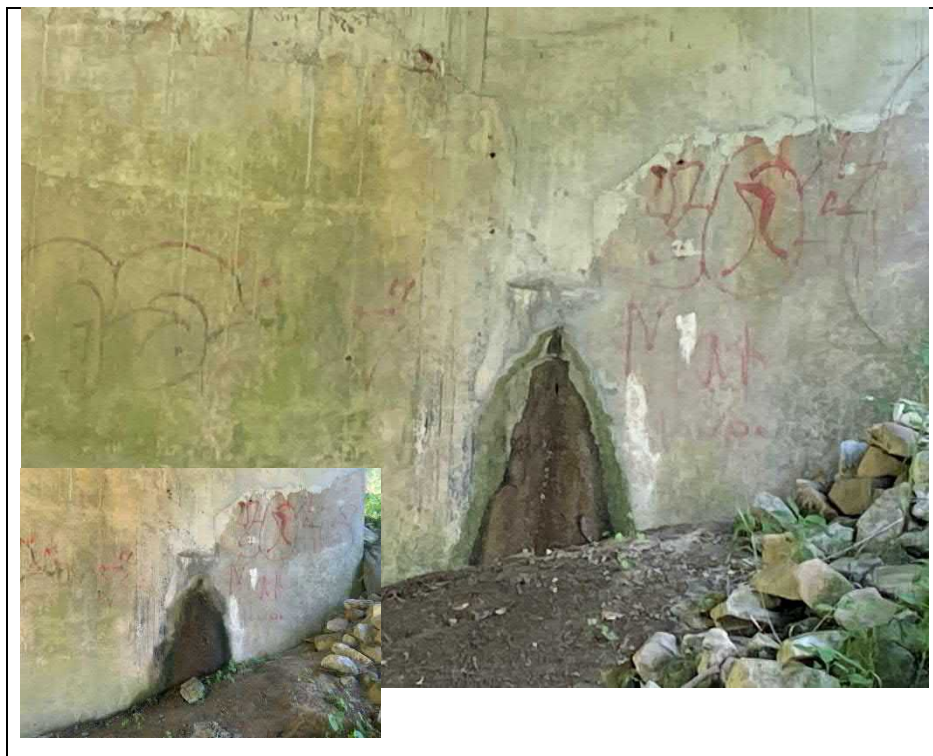
Photograph 20: Medium crack with active wet areas and efflorescence at south abutment wall
