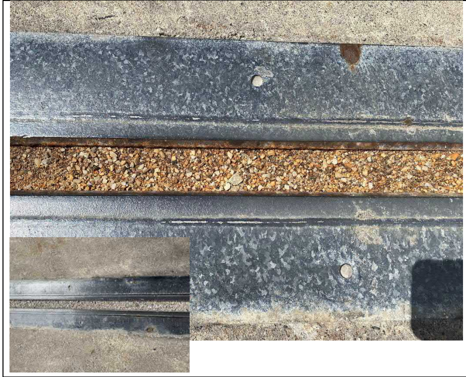
Photograph 7: Typical debris build up in expansion joints
