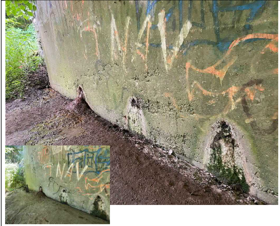
Photograph 17: Typical condition of wall drains on the south abutment wall and typical honeycombing
