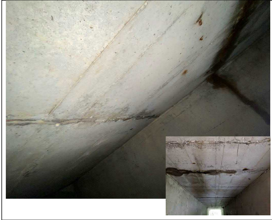
Photograph 13: Typical stained medium to wide cracks throughout the soffit (Looking Northwest)
