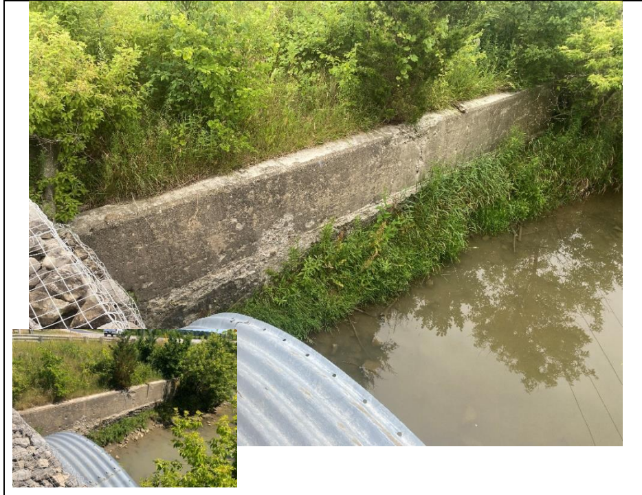
Photograph 17: Deterioration along the retaining wall at the southeast embankment consisted of medium spalling, severe scaling, pop outs and severe honeycombing along the bottom of the wall
