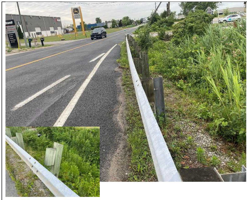
Photograph 8: Settled, rotated post of railing system at the northeast quadrant of structure (Looking Northeast)
