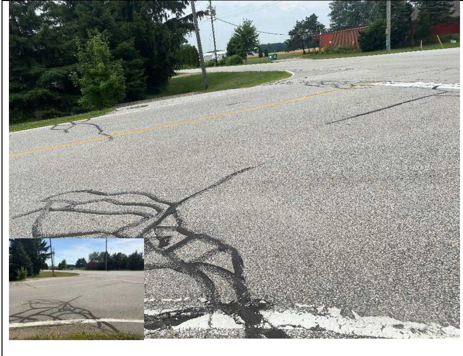
Photograph 3: Sealed map cracking on the Wearing surface at the east approach (Looking South)
