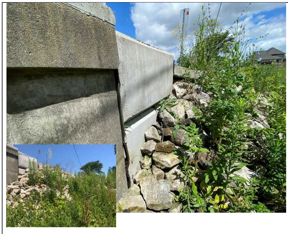
Photograph 10: New precast block retaining wall and slope protection at northeast embankment (Looking West)
