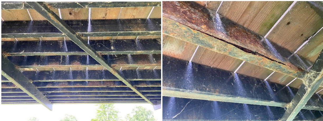
(a) Typical condition of the floor system with light corrosion and coating failure across all members.
