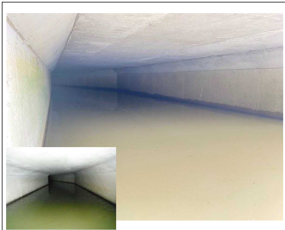
Photograph 10: North end of barrel (Looking South). Note: Picture from 2016. Barrel access is deemed Confined Space Entry
