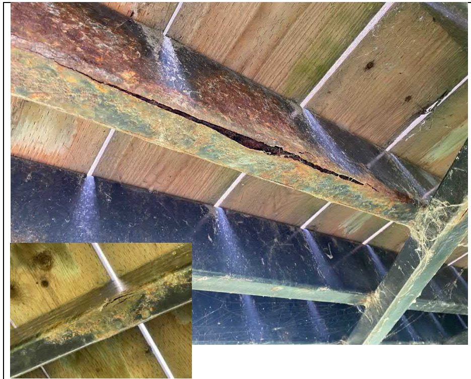
Photograph 12: Perforation observed on one stringer member
