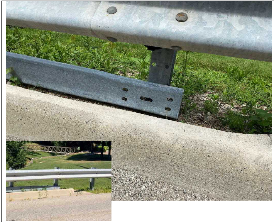
Photograph 13: Missing bolt(s) at bottom of northwest guardrail
