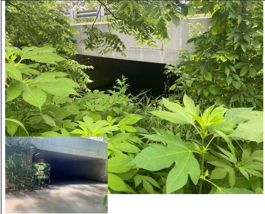
Photograph 7: East elevation with typical cracking with efflorescence at the headwalls
