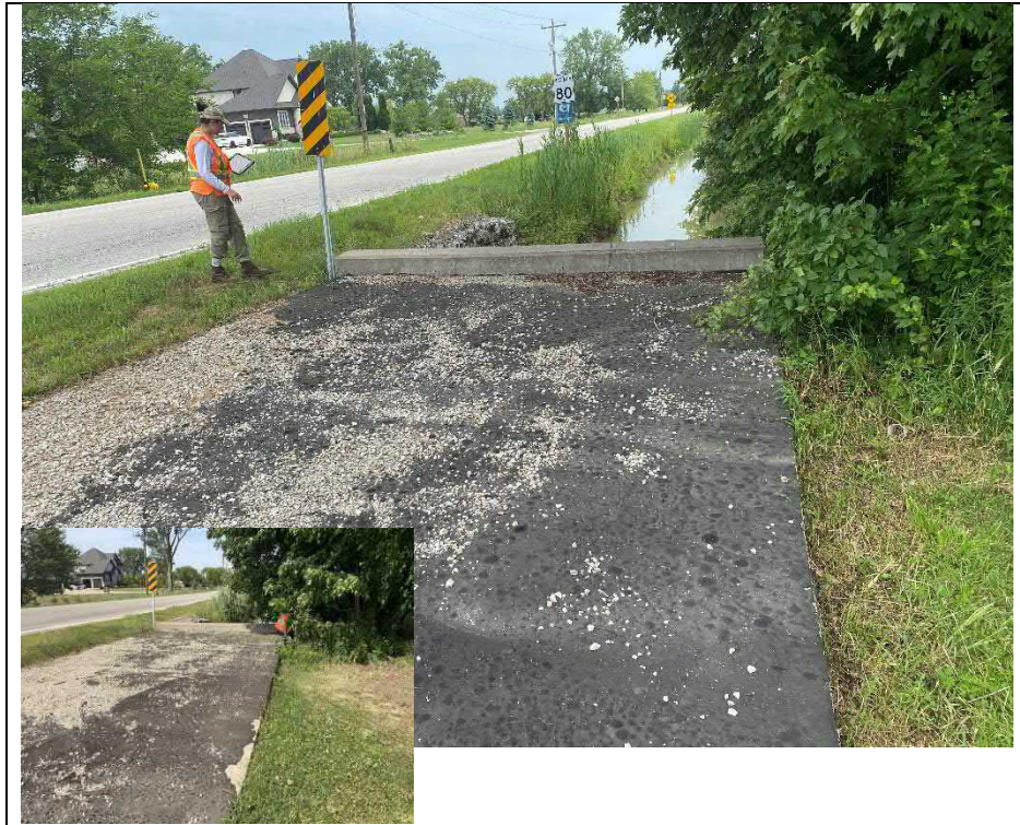
Photograph 7: Exposed waterproofing deterioration on north side of structure
