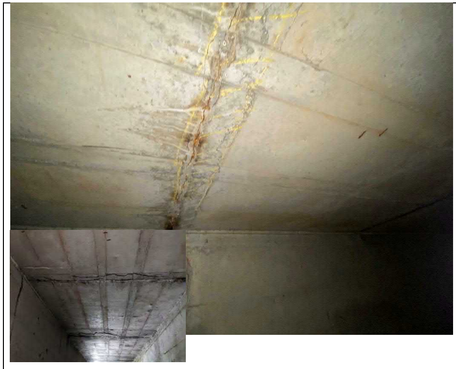
Photograph 14: Cracks extending from the culvert soffit to the abutments
