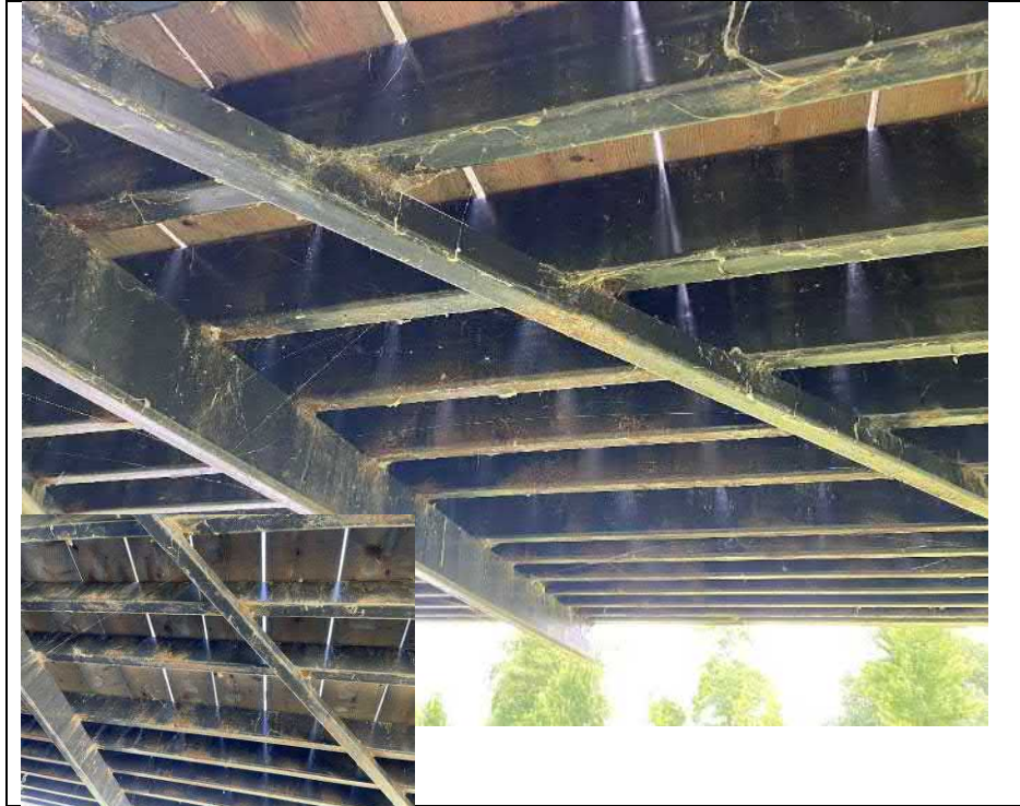
Photograph 13: Typical corrosion and coating failure of all members in the floor system
