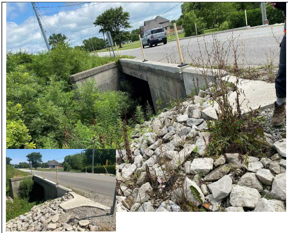
Photograph 4: Concrete spillway, precast block retaining wall and raised curb at southwest quadrant of structure (Looking North)
