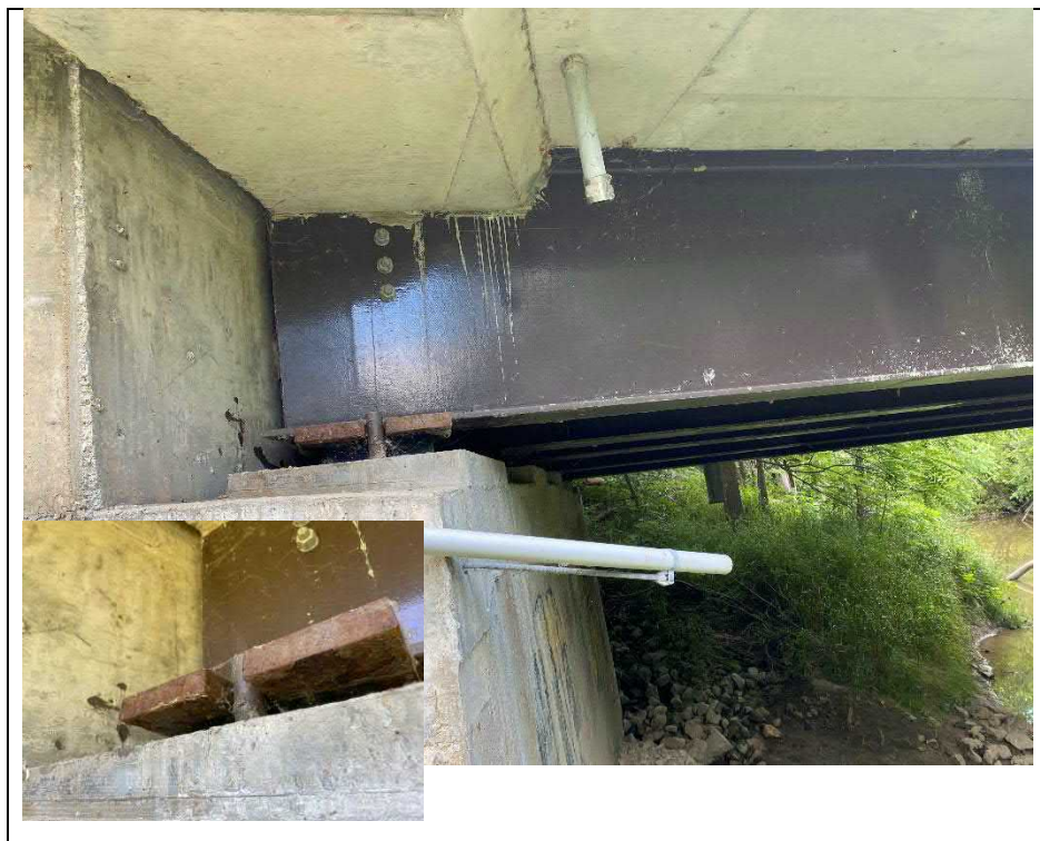
Photograph 18: Shoe plate corrosion at north abutment wall
