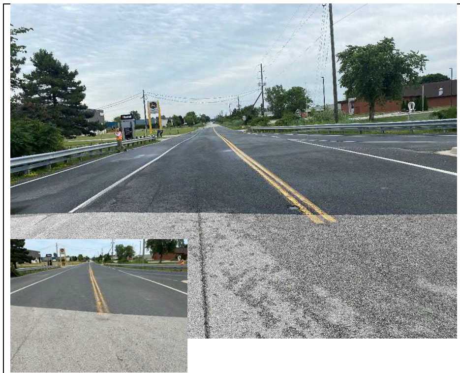
Photograph 4: Centreline of the road wearing surface approximately at mid span of the structure
