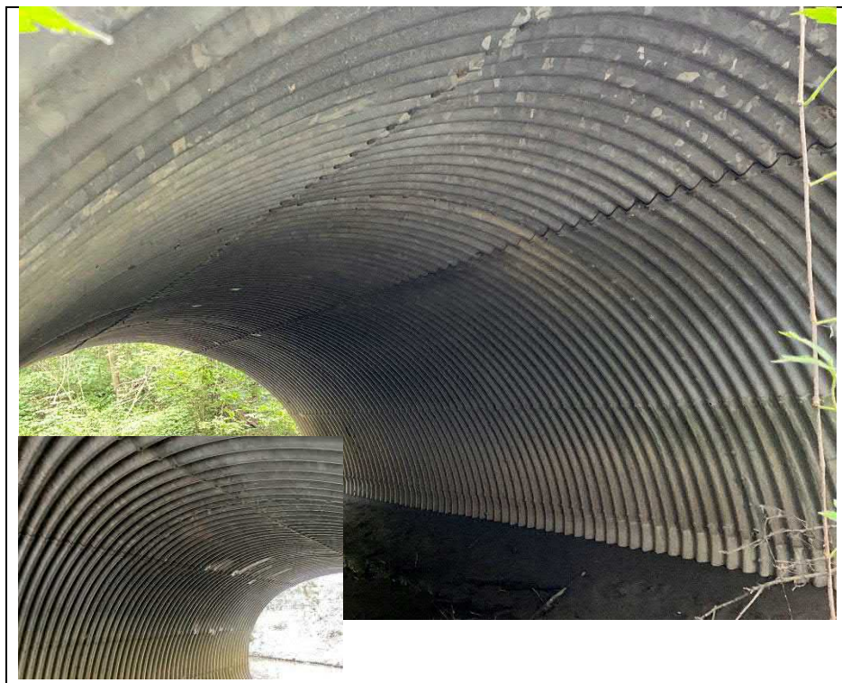
Photograph 10: Typical condition of culvert barrel soffit
