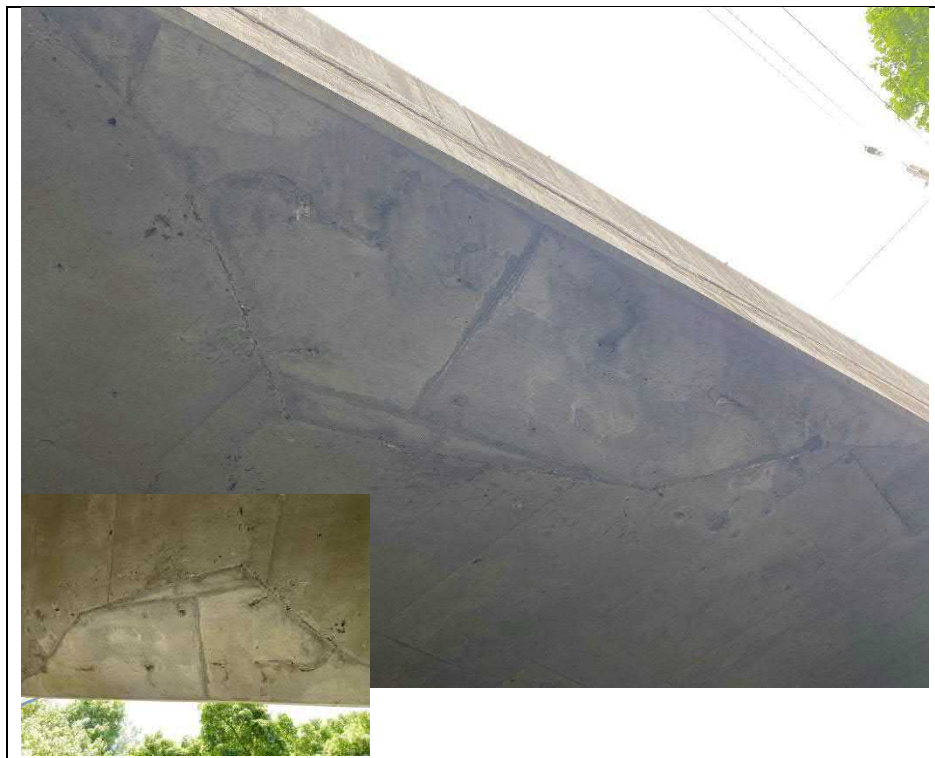
Photograph 18: Former wet staining and efflorescence on west edge of soffit (Rehab in 2016)
