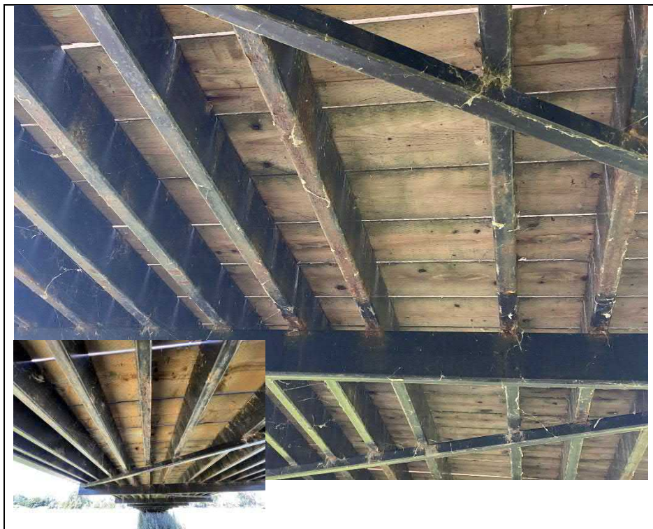
Photograph 10: Typical coating failure and light to medium corrosion throughout all stringers
