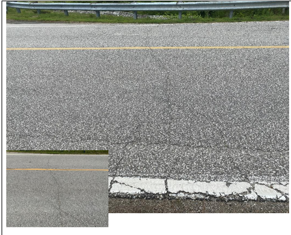
Photograph 3: Wide transverse cracking (Looking North)
