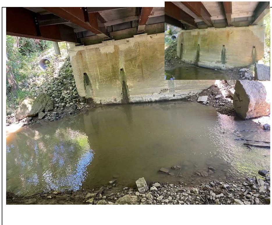
Photograph 14: Wall drains and erosion at footing at east abutment (Looking East)
