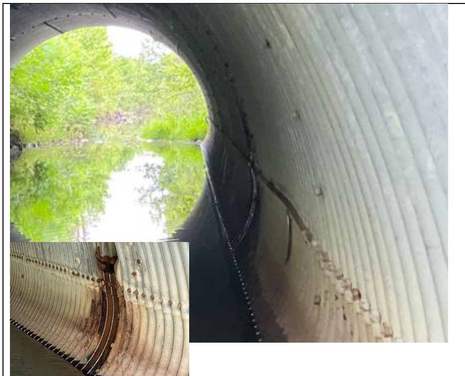
Photograph 14: Severe corrosion below inlet pipe at west wall
