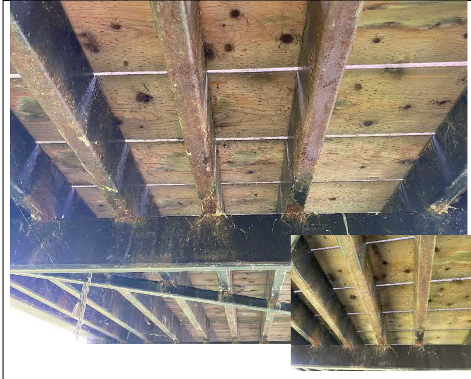
Photograph 9: Typical severe corrosion at stringer to floor beam weld locations
