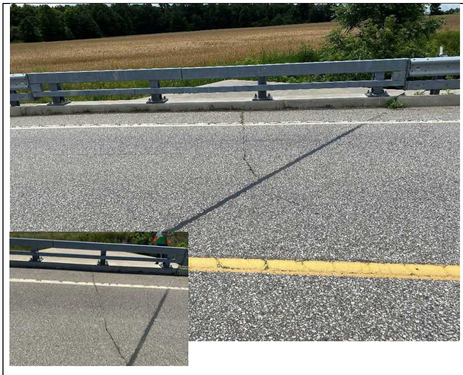
Photograph 4: Typical condition of barrier and wearing surface over the structure with medium transverse crack (Looking South)
