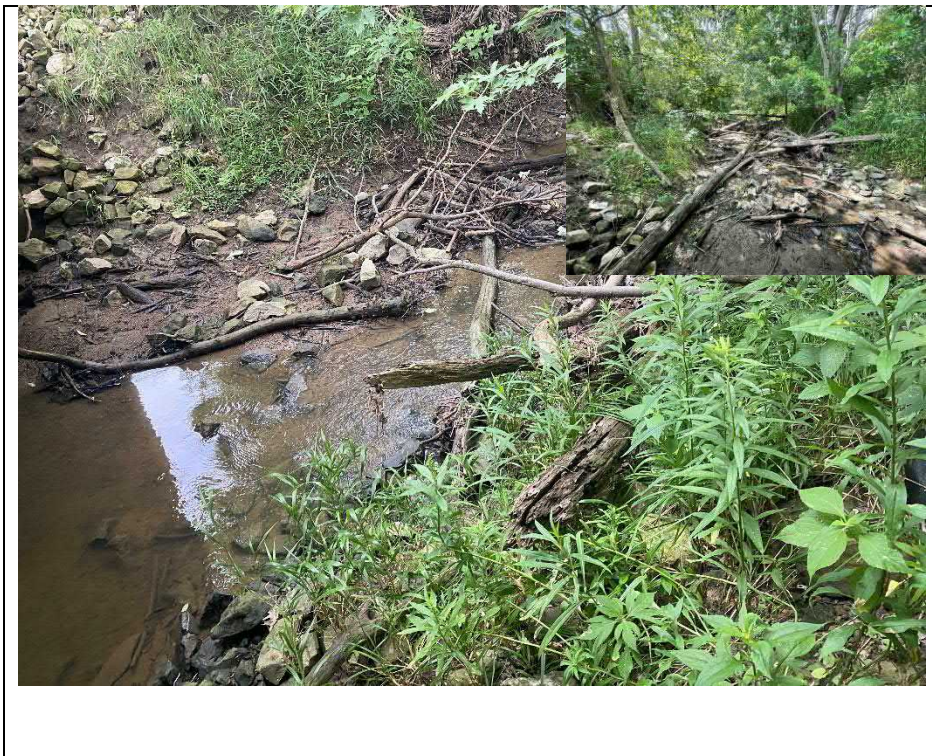
Photograph 14: Watercourse and south-west embankment with debris impeding flow
