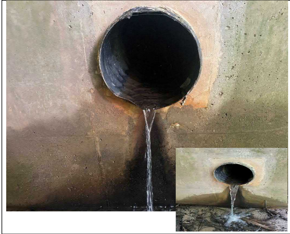
Photograph 9: South abutment wall near west extent of structure, HDPE outlet with corrosion staining beneath (Looking South)
