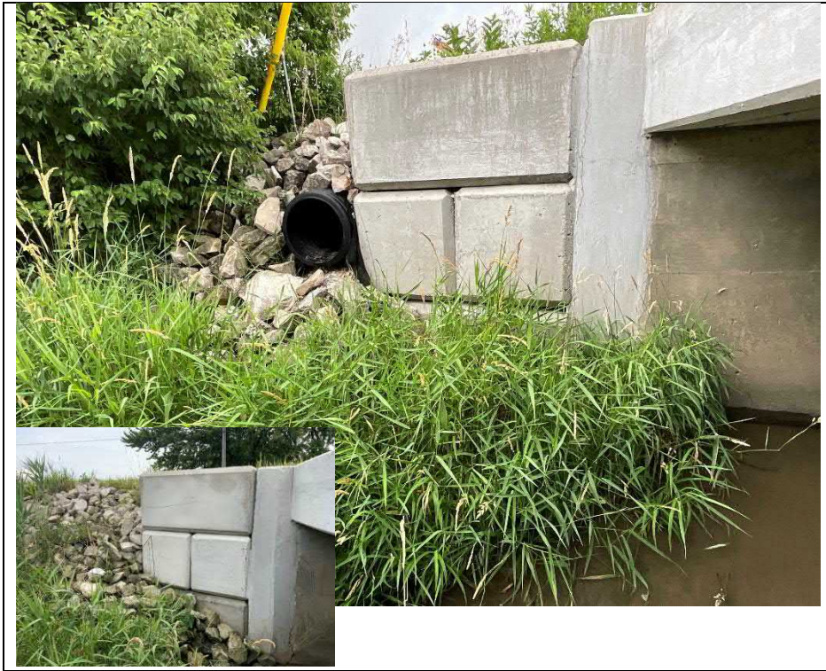
Photograph 11: Typical Precast block retaining walls, rip rap and sub drains at embankments
