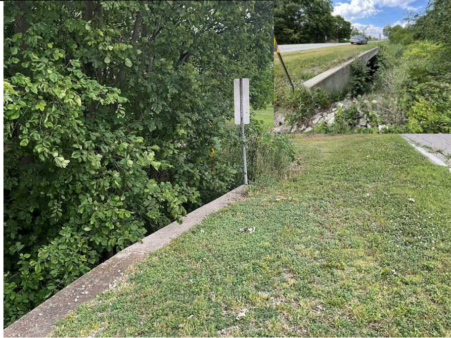
Photograph 5: Severe erosion of the shoulder at the southeast embankment
