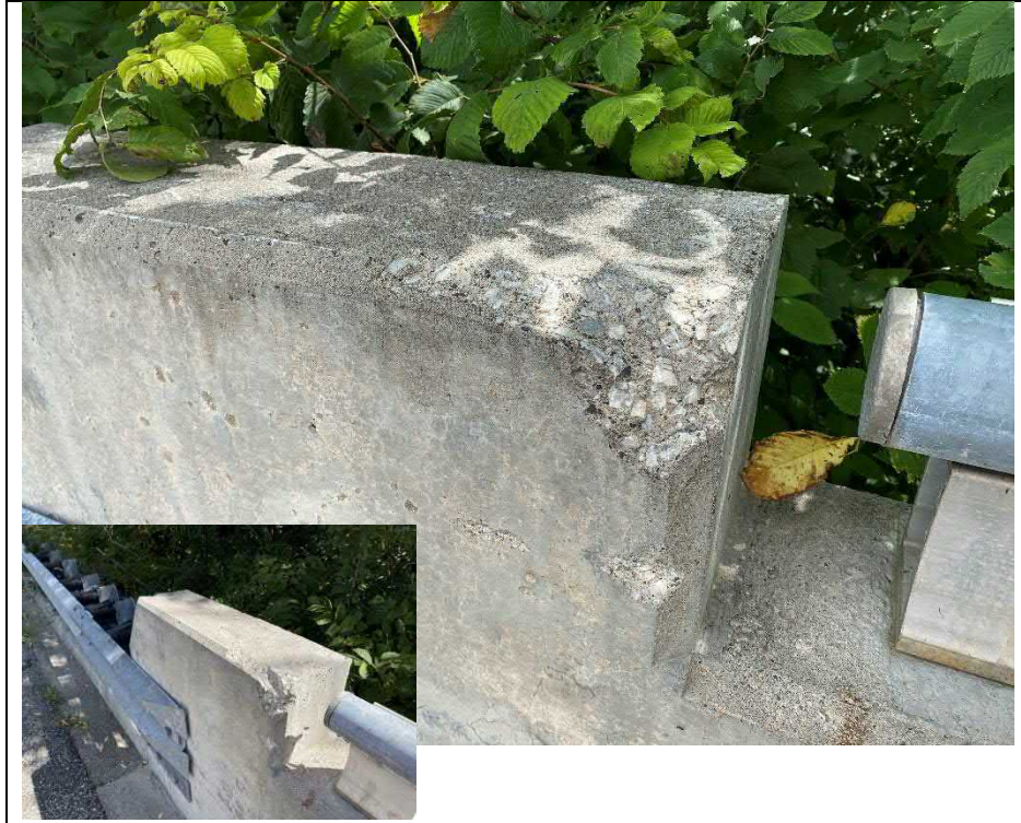
Photograph 11: Light spall on north east end wall
