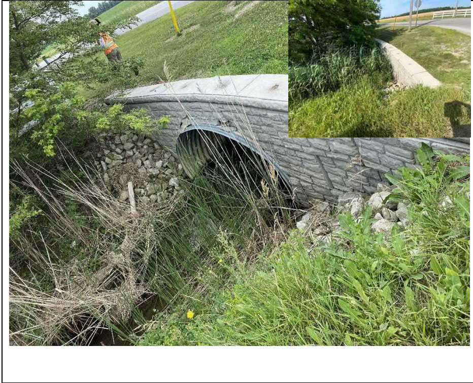
Photograph 5: West elevation with excessive vegetation (Looking North)
