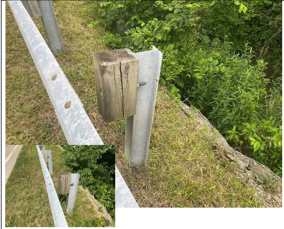
Photograph 5: Guide rail on southeast quadrant of structure with detached post
