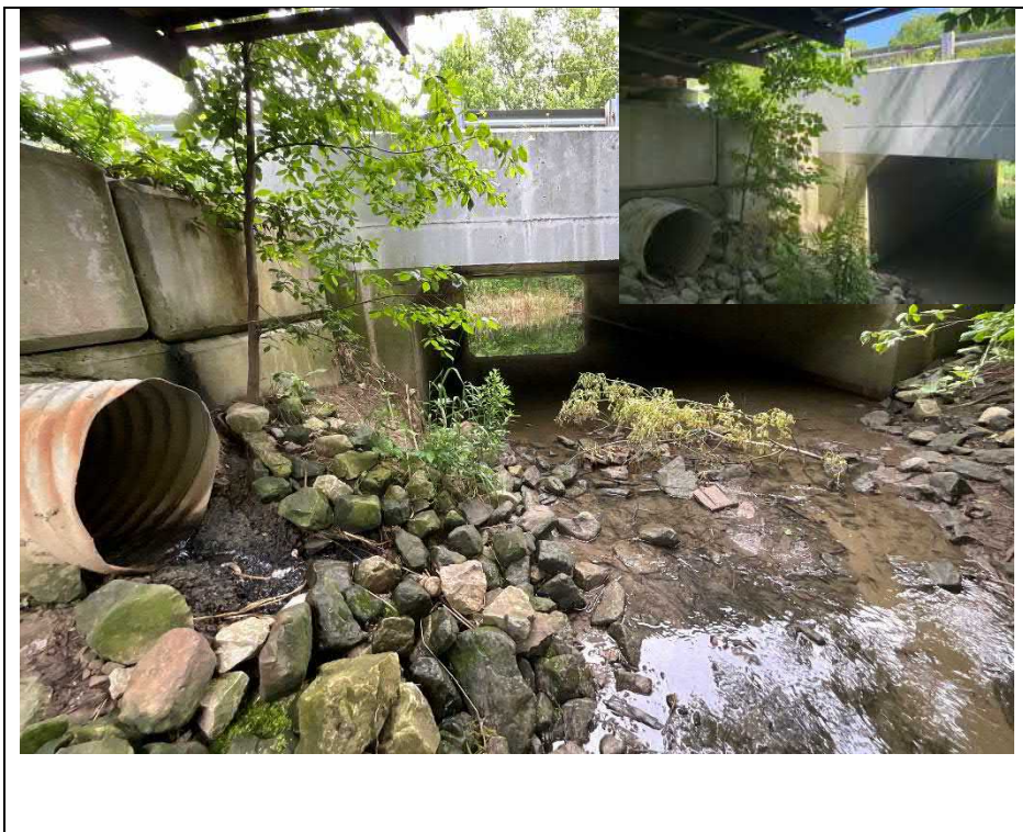
Photograph 16: C.S.P outlet, retaining structure, pedestrian bridge and abutment at west side of structure (Looking North)
