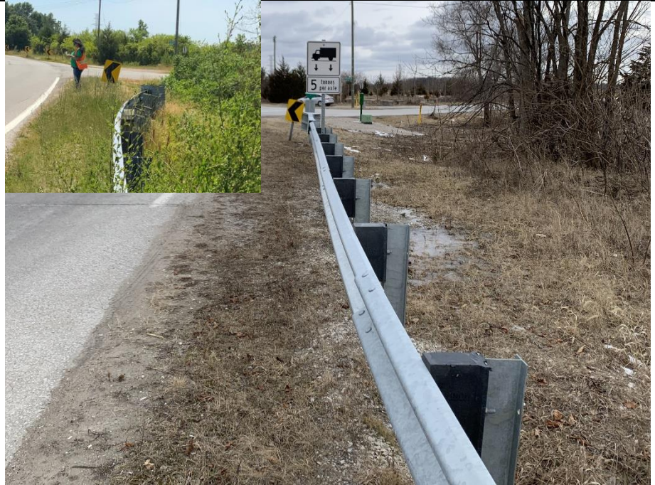
Photograph 5: Load limit sign and new guide rail section at the northwest end
