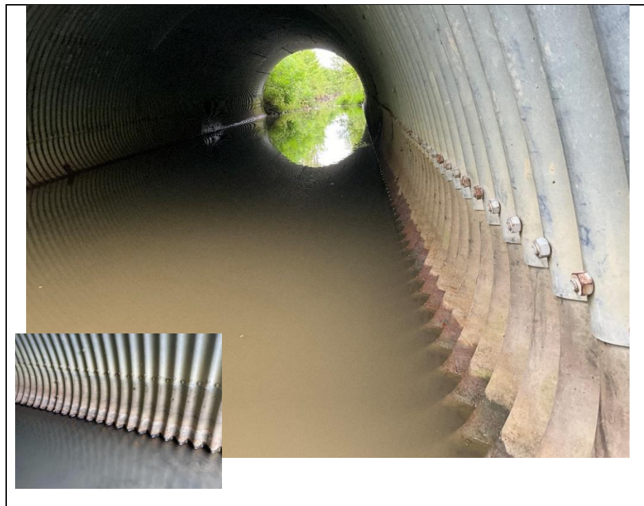
Photograph 12: Typical loss of coating and light to medium corrosion along the water line
