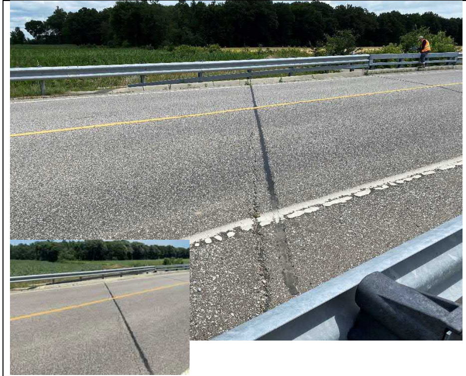
Photograph 3: Typical condition of wearing surface at approaches (Looking East)
