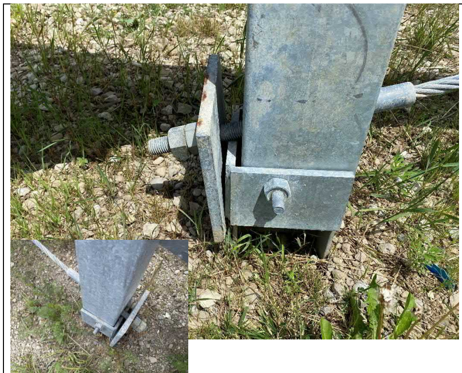
Photograph 6: Guiderrail cable anchorage observed to be loose at all 4 quadrants
