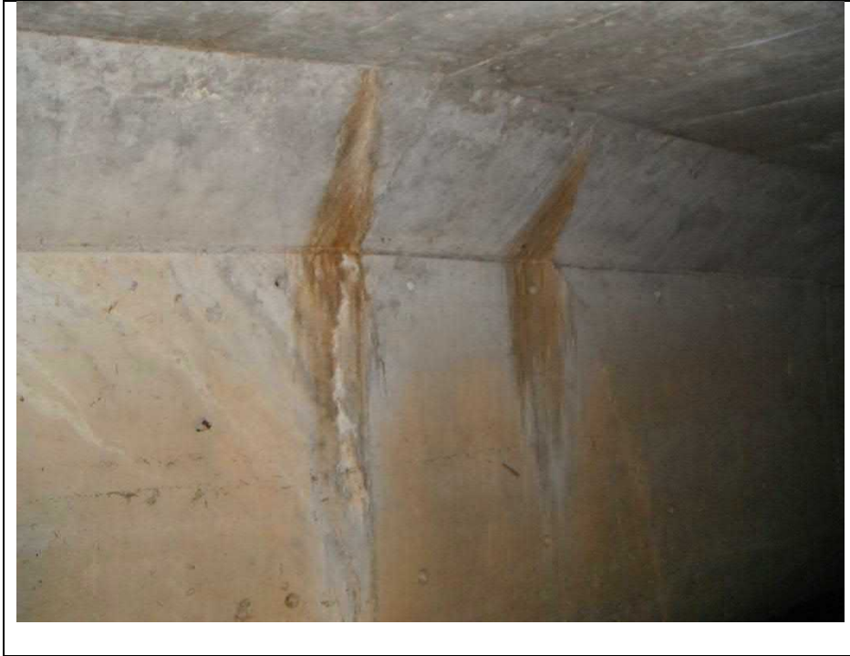
Photograph 11: Two vertical cracks at the east barrel wall. Note: Picture from 2016. Barrel access is deemed Confined Space Entry
