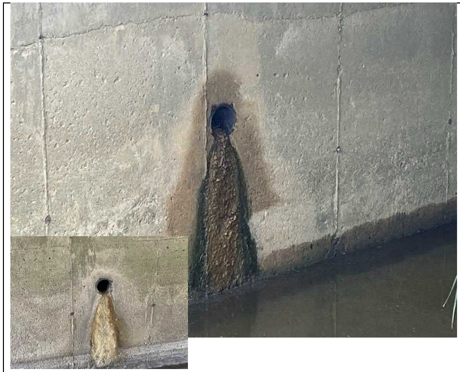
Photograph 12: Typical condition of wall drains in culvert barrel with wet staining and efflorescence
