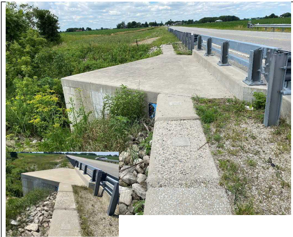
Photograph 18: Severe scaling on top of one precast retaining wall block at southeast side of culvert
