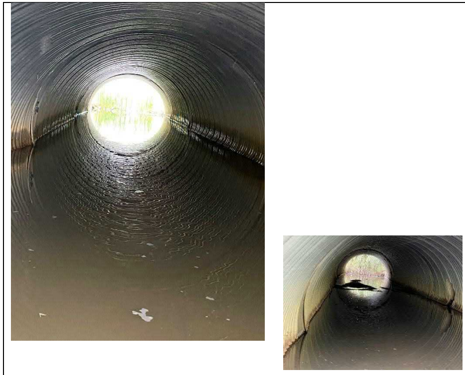
Photograph 8: Typical transverse joint deformation and light to medium corrosion along the waterline
