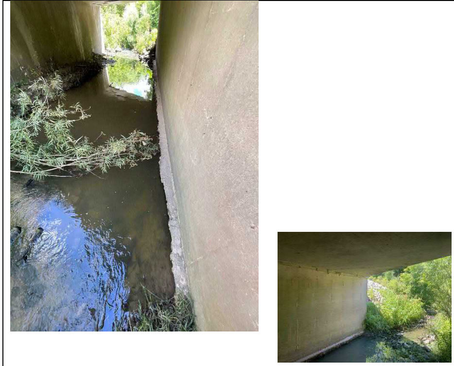
Photograph 9: Scour and concrete erosion at south abutment footings (typ.)
