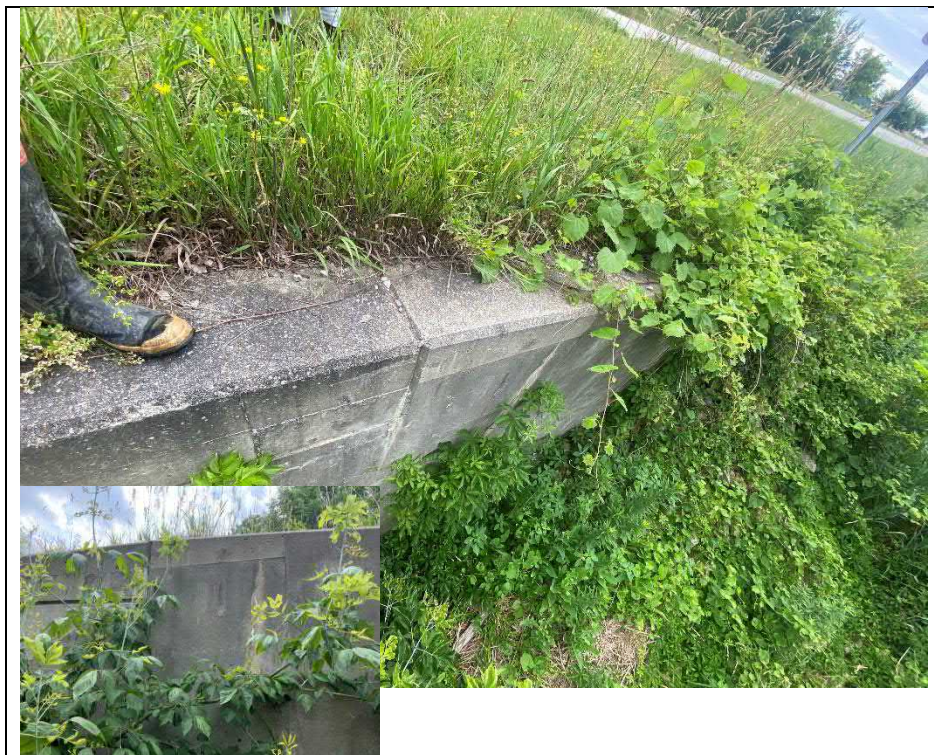
Photograph 10: North-west wing wall with efflorescent-stained vertical crack
