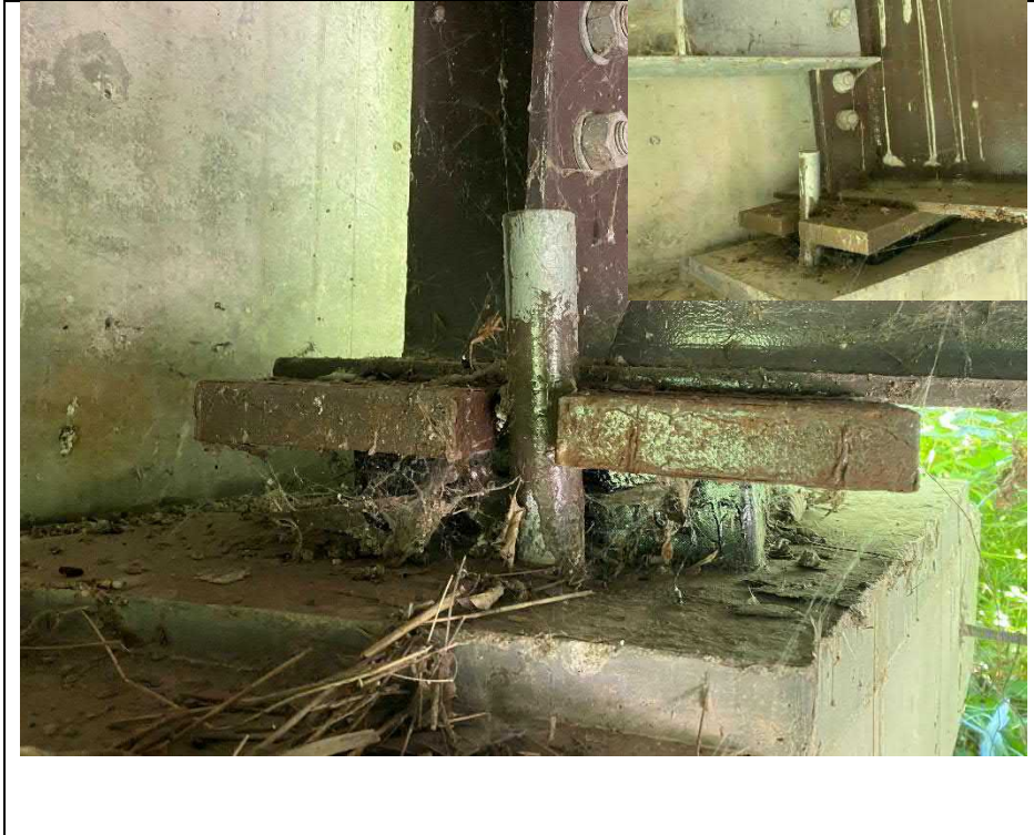
Photograph 13: Misaligned anchor rod at abutment bearings (typ.)
