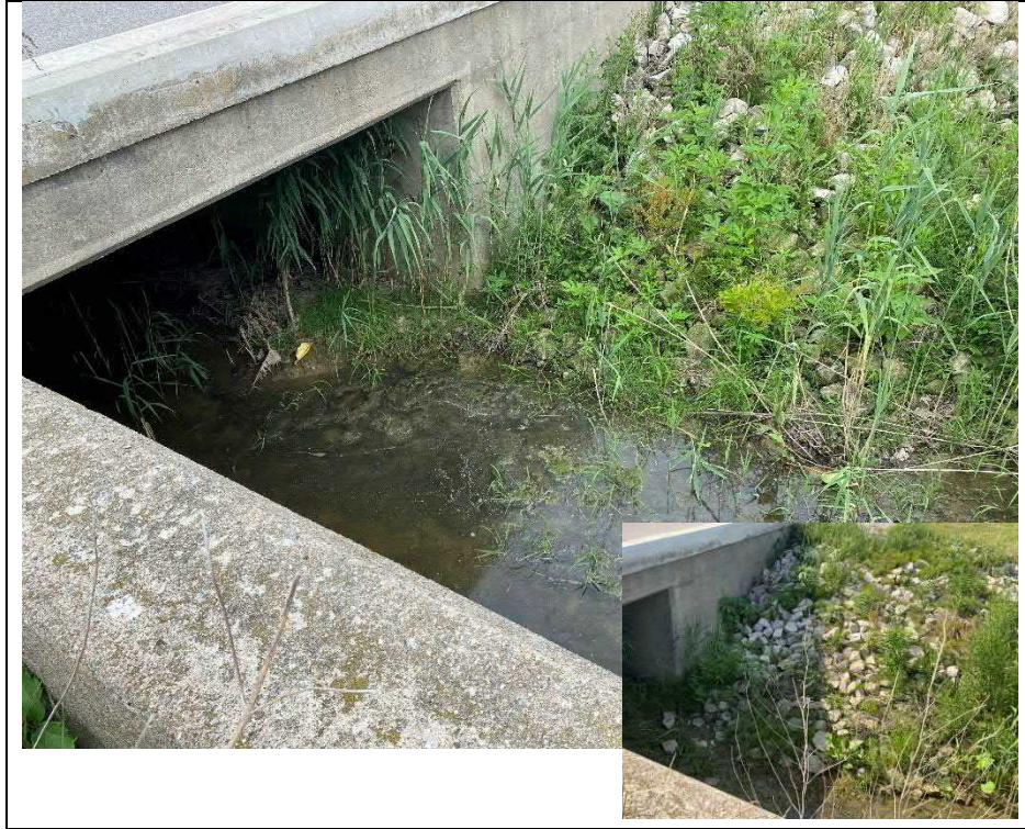
Photograph 13: Watercourse on east side of structure, and slope protection rip-rap (Looking North)
