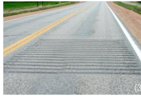
Rumble strip Vertical deflection; Small bumps in the roadway surface causing vibration in automobiles
