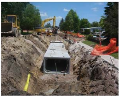
Increased sewer conveyance
