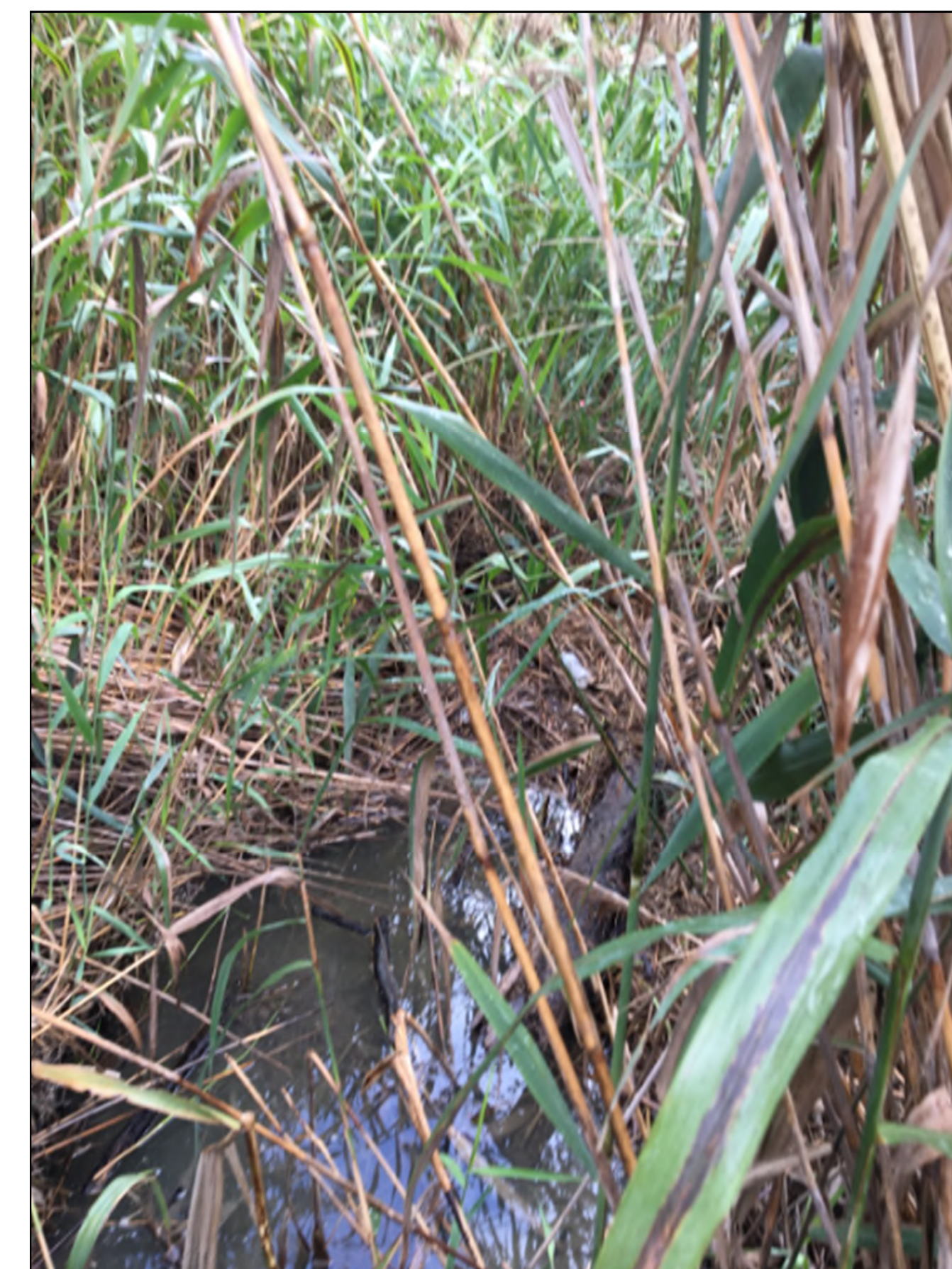
PARTIAL BLOCKAGE IN DRAIN
